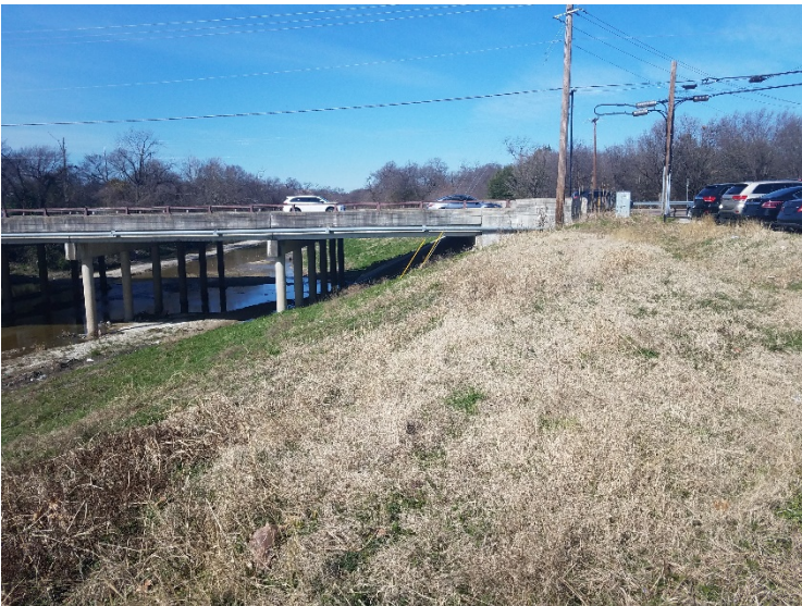
Photograph 11 – Graded creek bank passing under Centerville Road bridge within Northern APE, view to the northwest.
