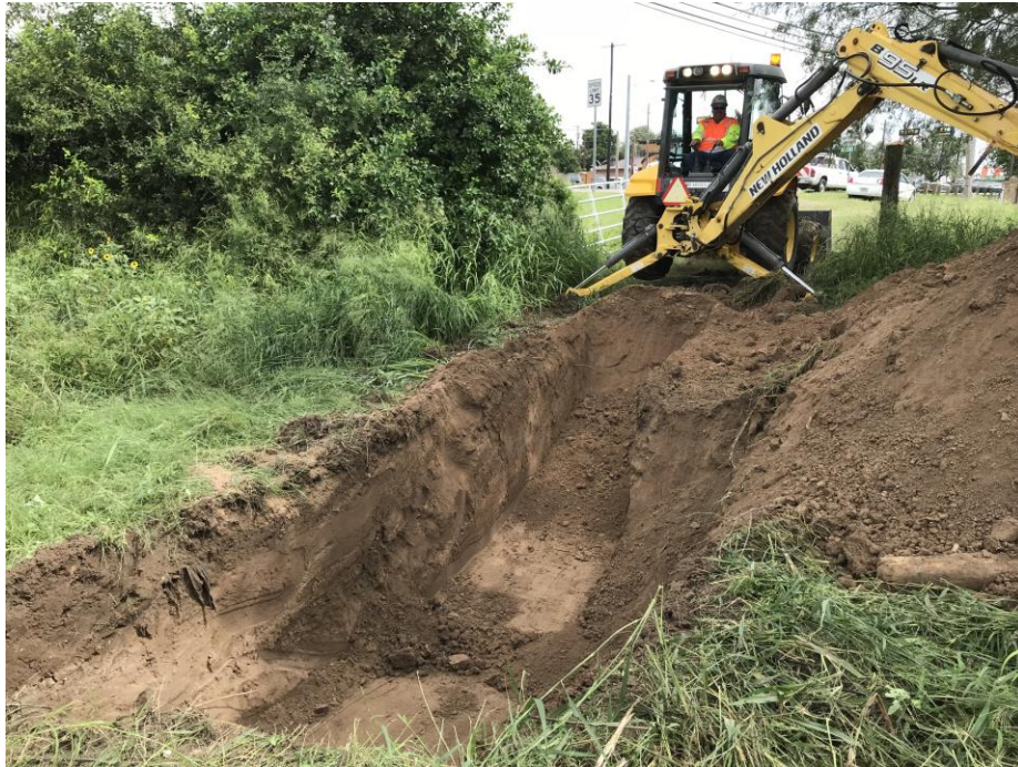
Trench 1 at Arroyo Roma Access Drive Project Area within Parcel 16(looking northeast).
