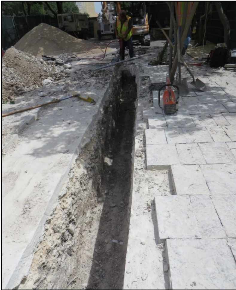
Figure 4-5. Use of the impact hammer. Portion of the Phase II trench, facing south.
