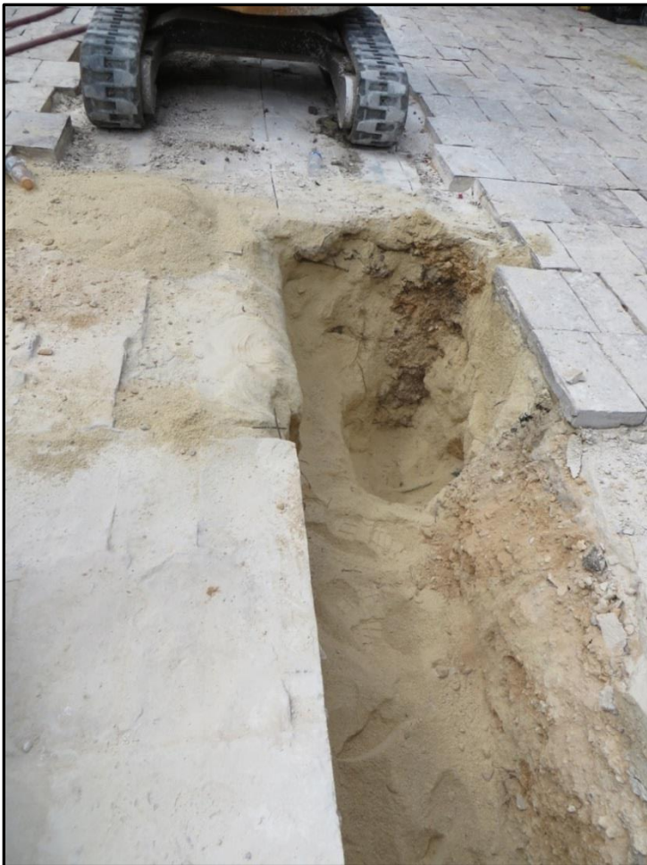
Figure 4-6. Phase II trench showing sand and water line servicing the Spanish Governor's Palace.
