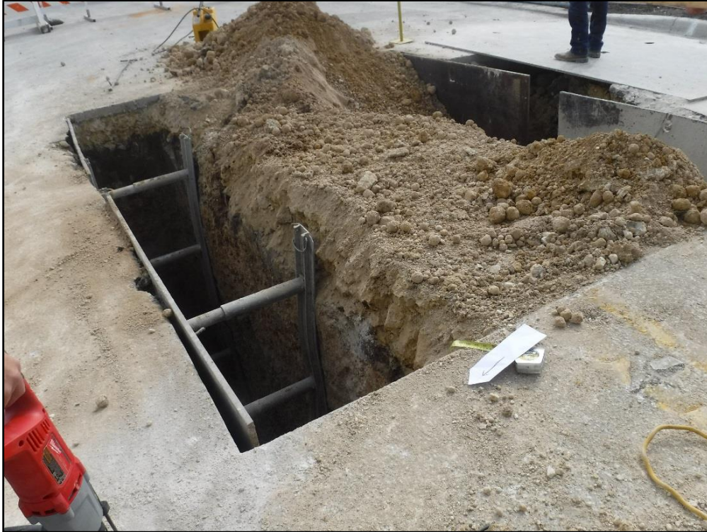
Figure 5-4. Overview of manhole pit excavation with shoring plates set along the northwestern and southeastern profiles, facing southeast.
