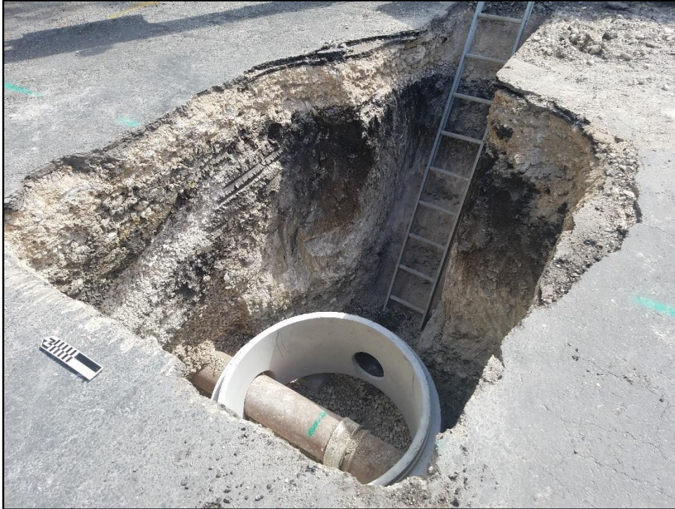
Figure 5-3. Installation of new sewer manhole at the junction of an existing SAWS sewer main, facing northeast.
