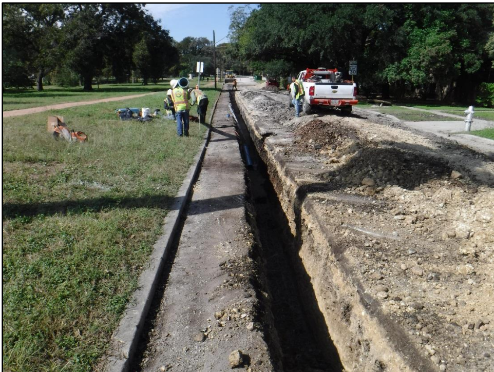
Figure 5-15. Overview of water main installations within the APE, facing west.
