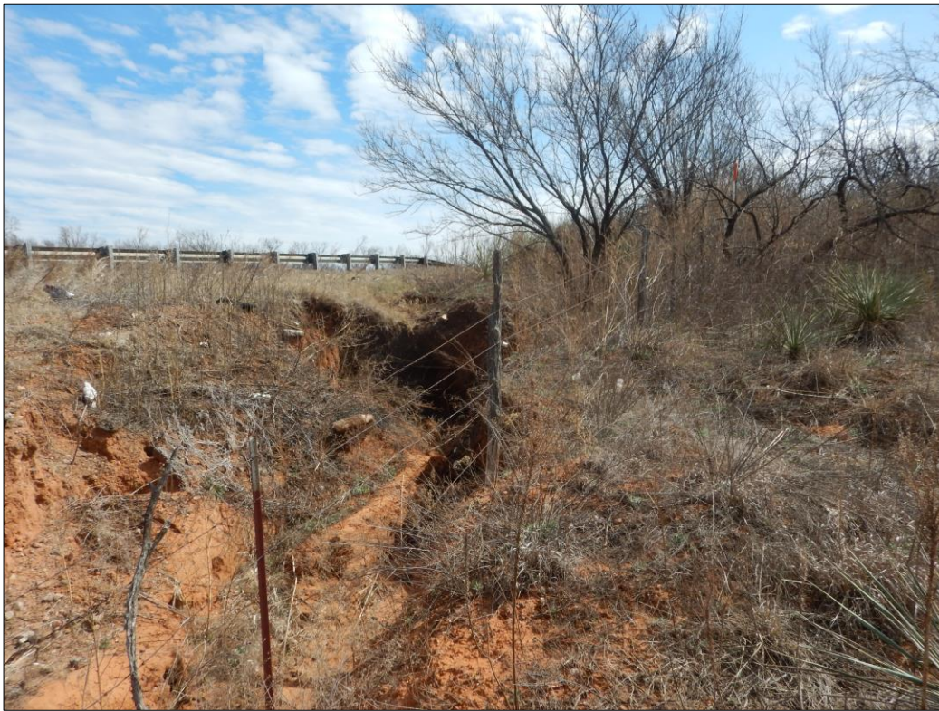
Figure 19: Terraforming and erosion south of US 287.
