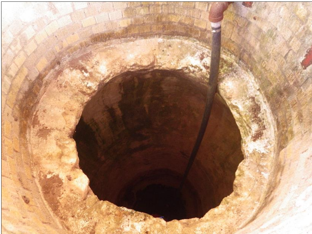
Figure 16. Cistern associated with the original Harbert Plantation; upper – cistern in front of barn, note the brick collar; lower – view inside the collar and cistern opening.
