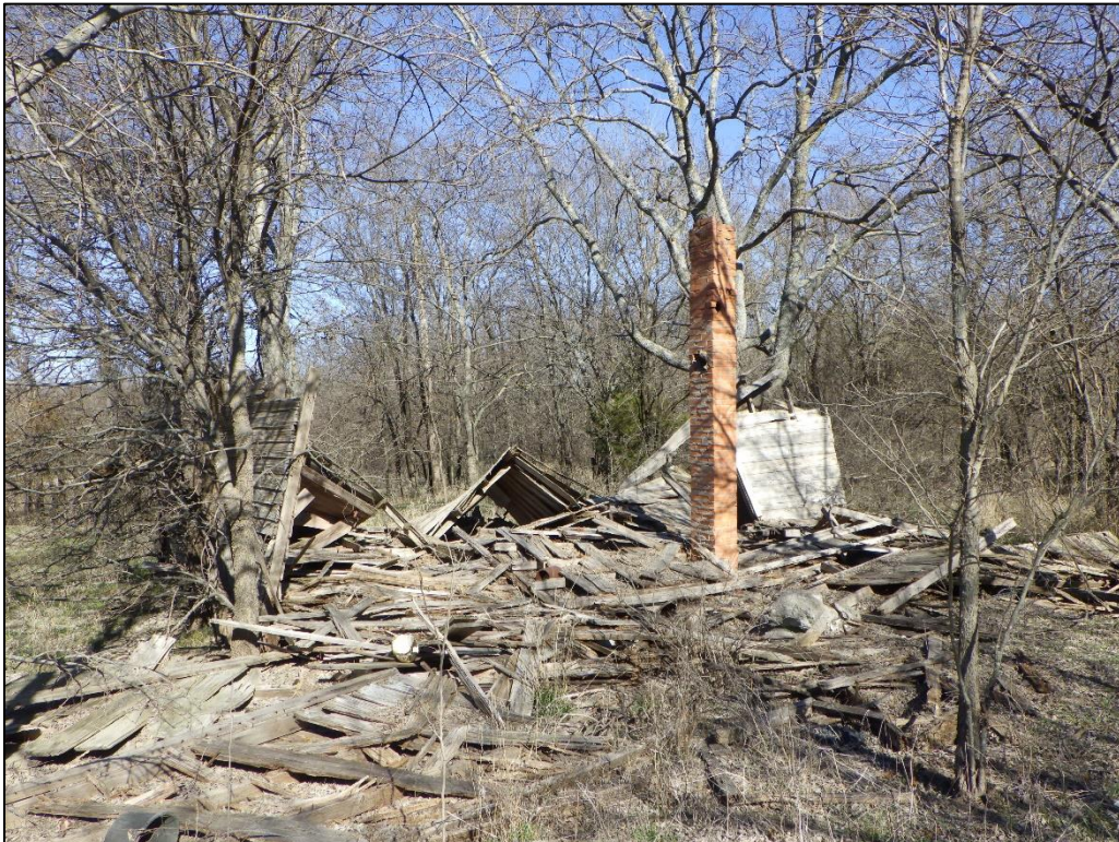
Figure 11. Collapsed pier and beam structure at 41COL328, facing northeast.
