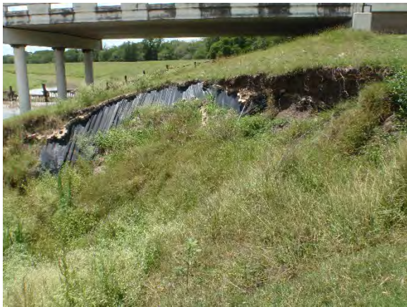
Figure 5-12. Overview of Workspace A APE with large erosional feature showing fill deposits located at Workspace A. View is to the north.
