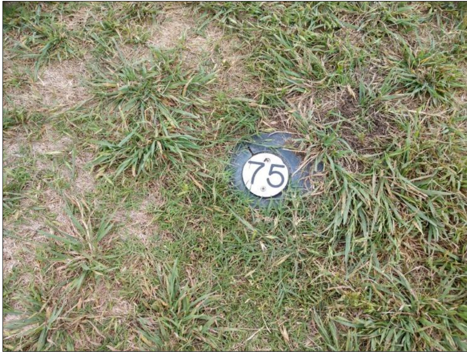
Figure 8. Sprinkler line within Disturbed Area 1.
