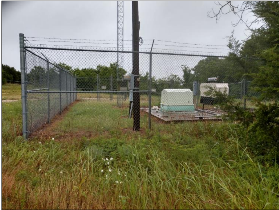
Figure 16. Utility substation in Disturbed Area 3.
