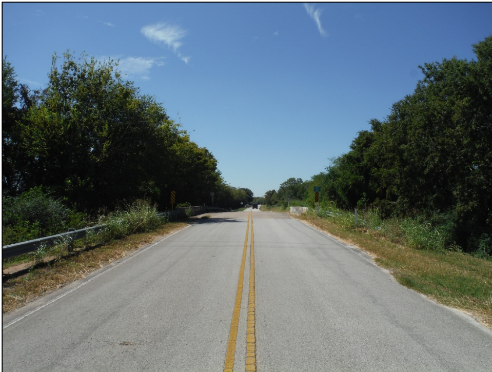
Figure 5-5. Overview of culvert and guard rails at Little Cypress Creek; facing west.
