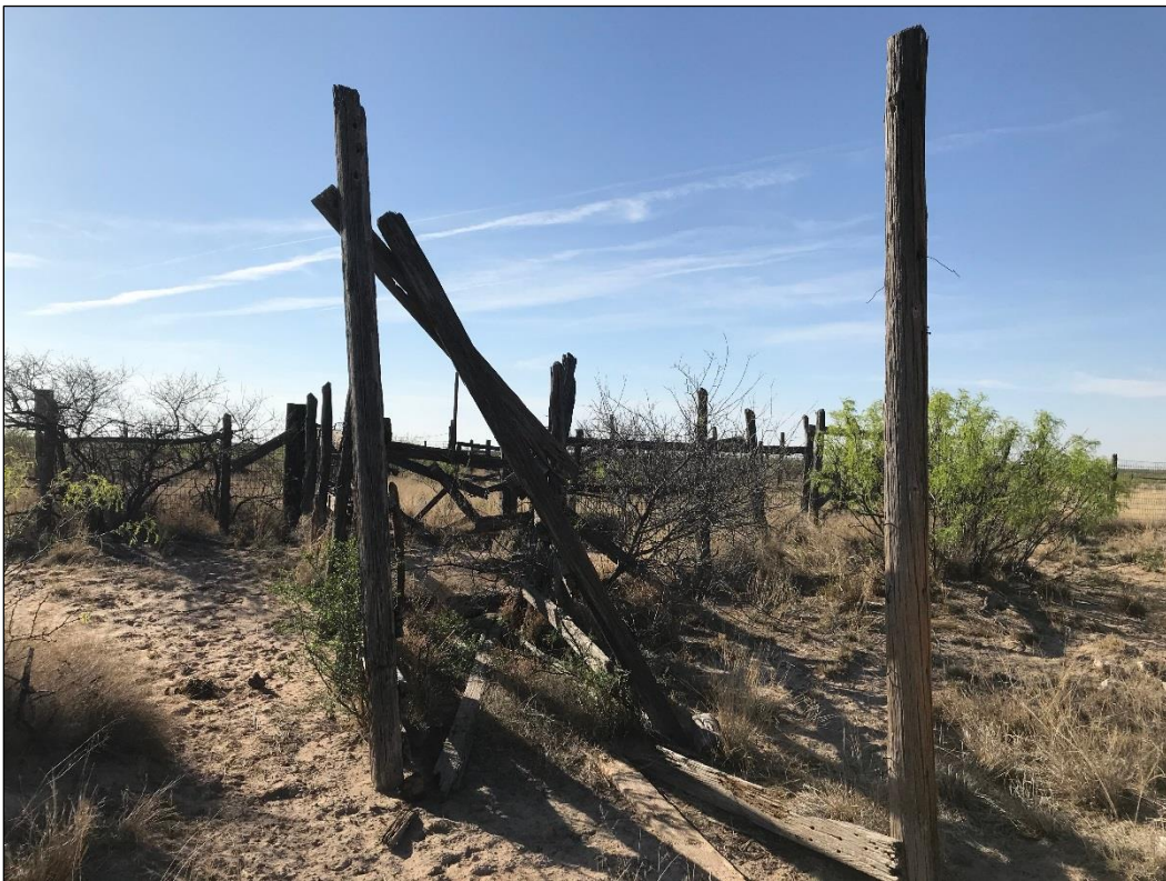
Figure 12. Second cattle chute at north end of dilapidated corral/pen at Site 41WK131, facing southeast.
