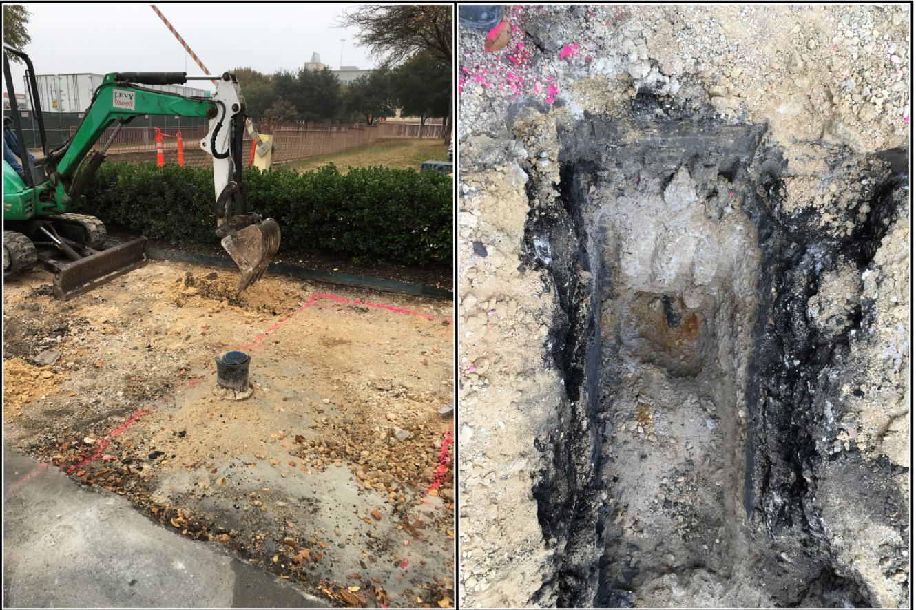
Figure 6-4. Excavation of Trench 3 on the south side of Buena Vista and S. Leona streets (left). The right image shows the trench with asphalt and flowable fill over an existing cast iron pipe.
