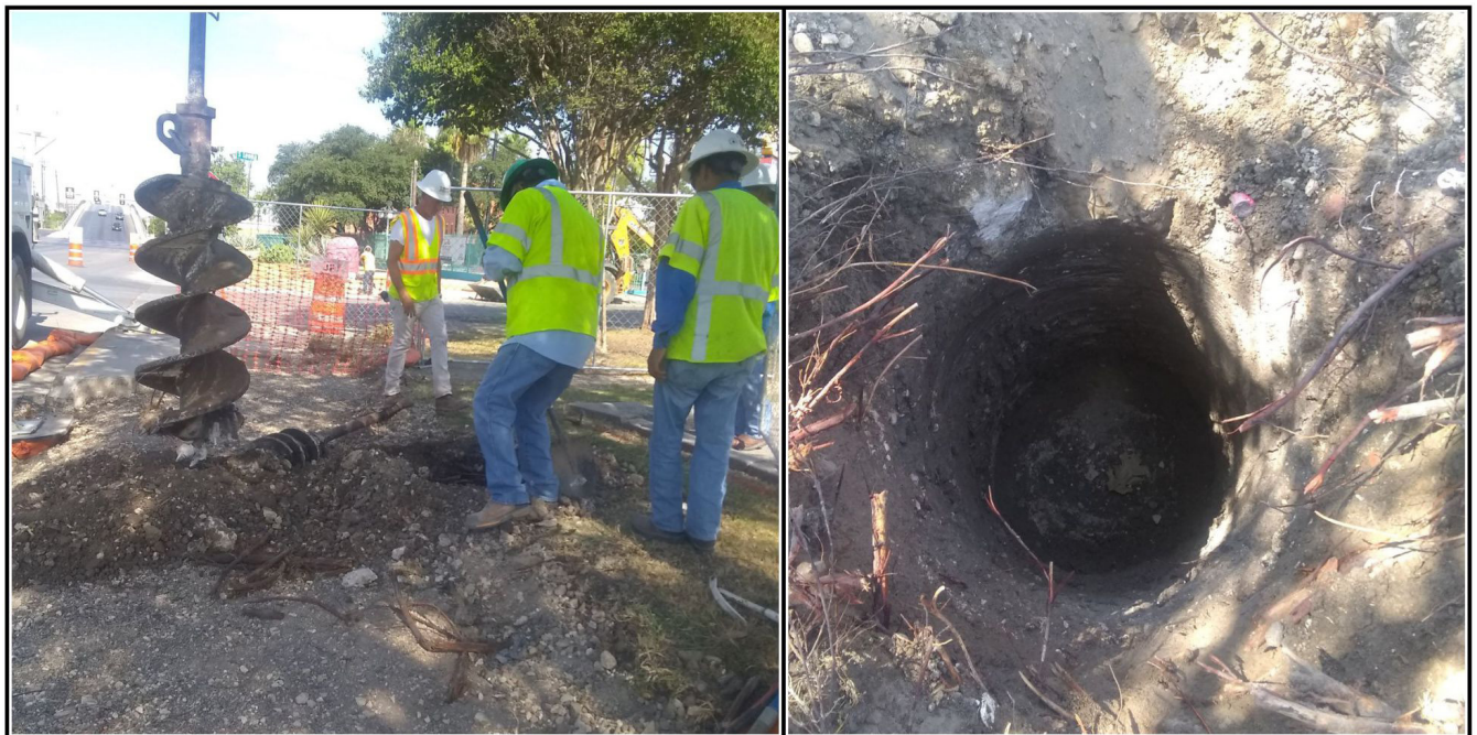
Figure 6-7. Auger excavation at S. Leona and Buena Vista streets (left). The image of the right shows concrete at 152.4 cm (5 ft.) below the surface.
