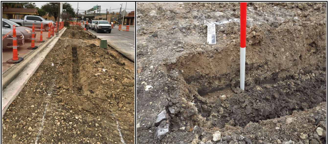
Figure 6-5. View to the west of the irrigation trench excavation with layout for planter boxes painted in white (left). Typical profile of irrigation wall view with construction fill to 25 cm (9.8 in.) below the grade followed by 5 cm (1.9 in.) of silty clay (right).
