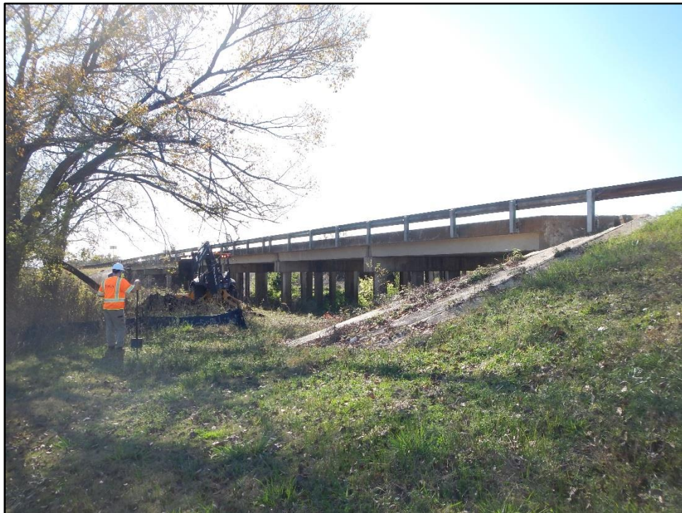
Figure 17. Overview of BHT01 excavation between the eastern side of the bridge and a buried AT&T fiber optic line within the existing ROW, facing southwest.
