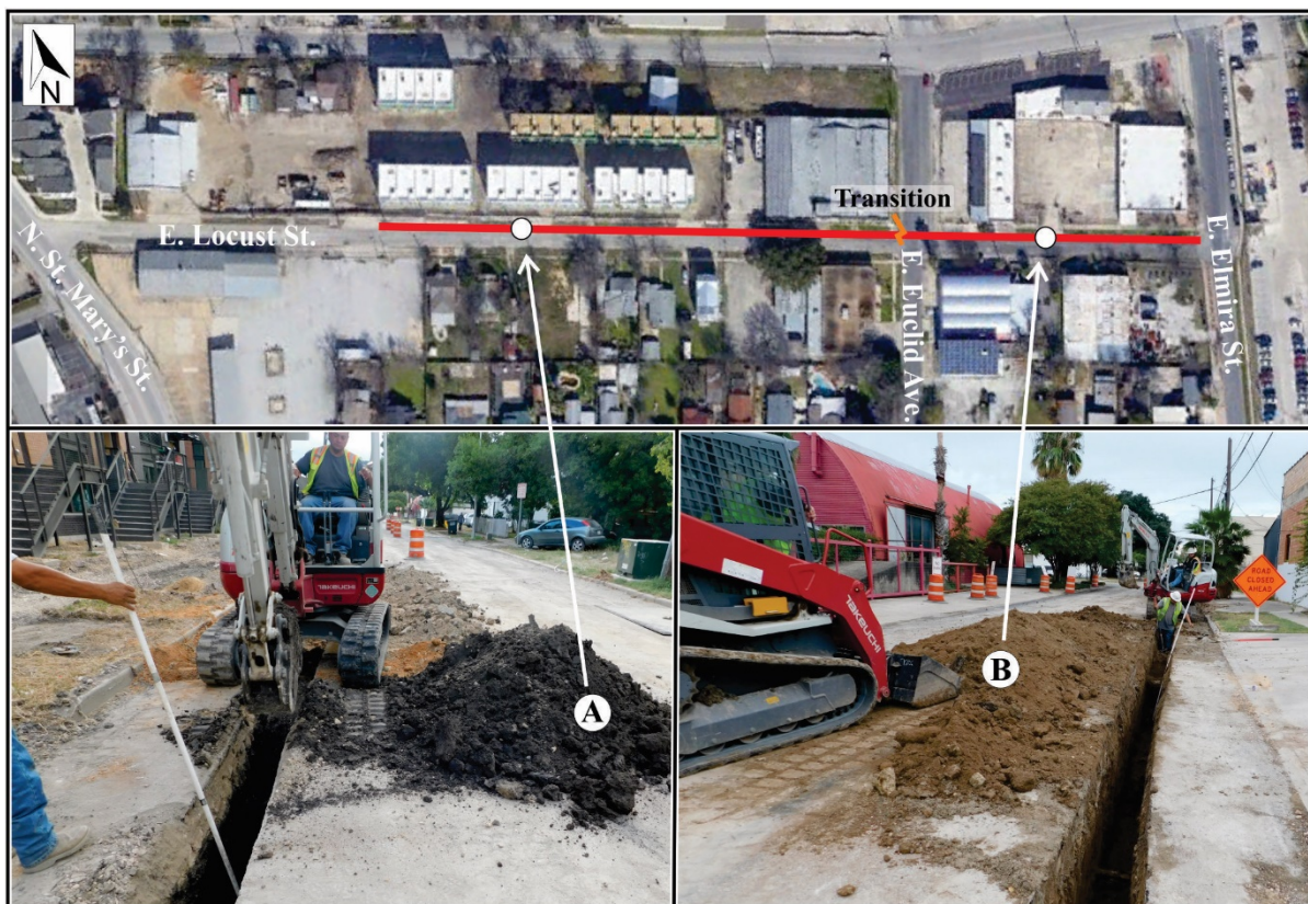
Figure 4-1. Excavated soil at west and east ends of the APE; transition at right of center.
