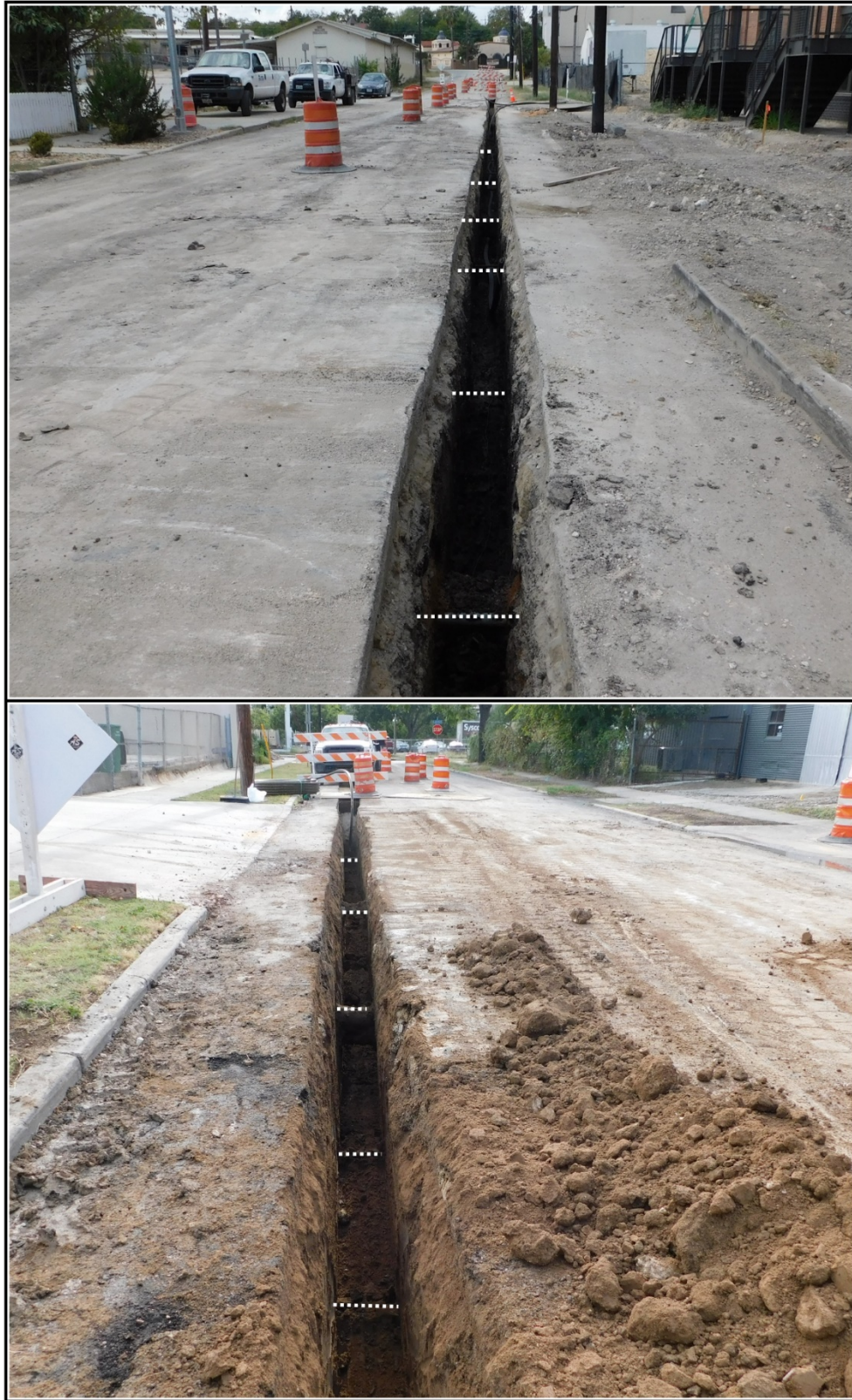
Figure 4-2. Trenching along west and east ends of the APE. Numerous utilities cross the trench and are highlighted by dashed lines (white).
