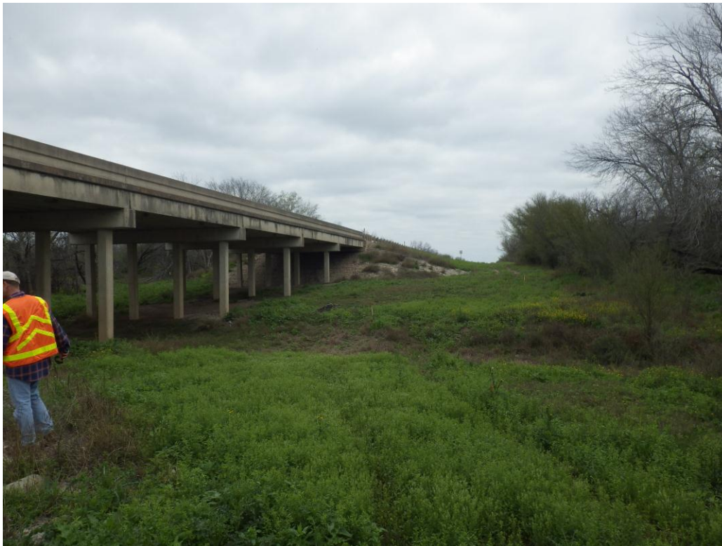
Figure 4. Mossy Slough Tributary Bridge at SH97 note shallow channel and fill section.
