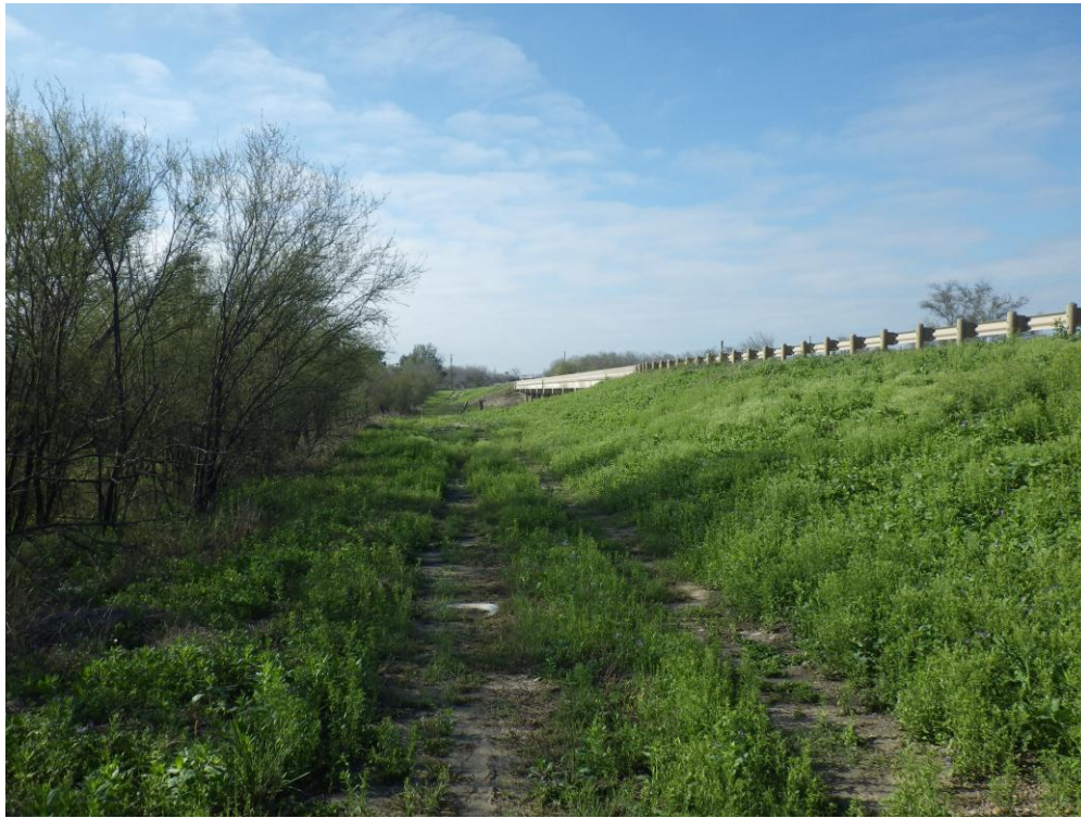
Figure 3. Fill section on northeast quadrant of the Frio River Bridge at SH97.
