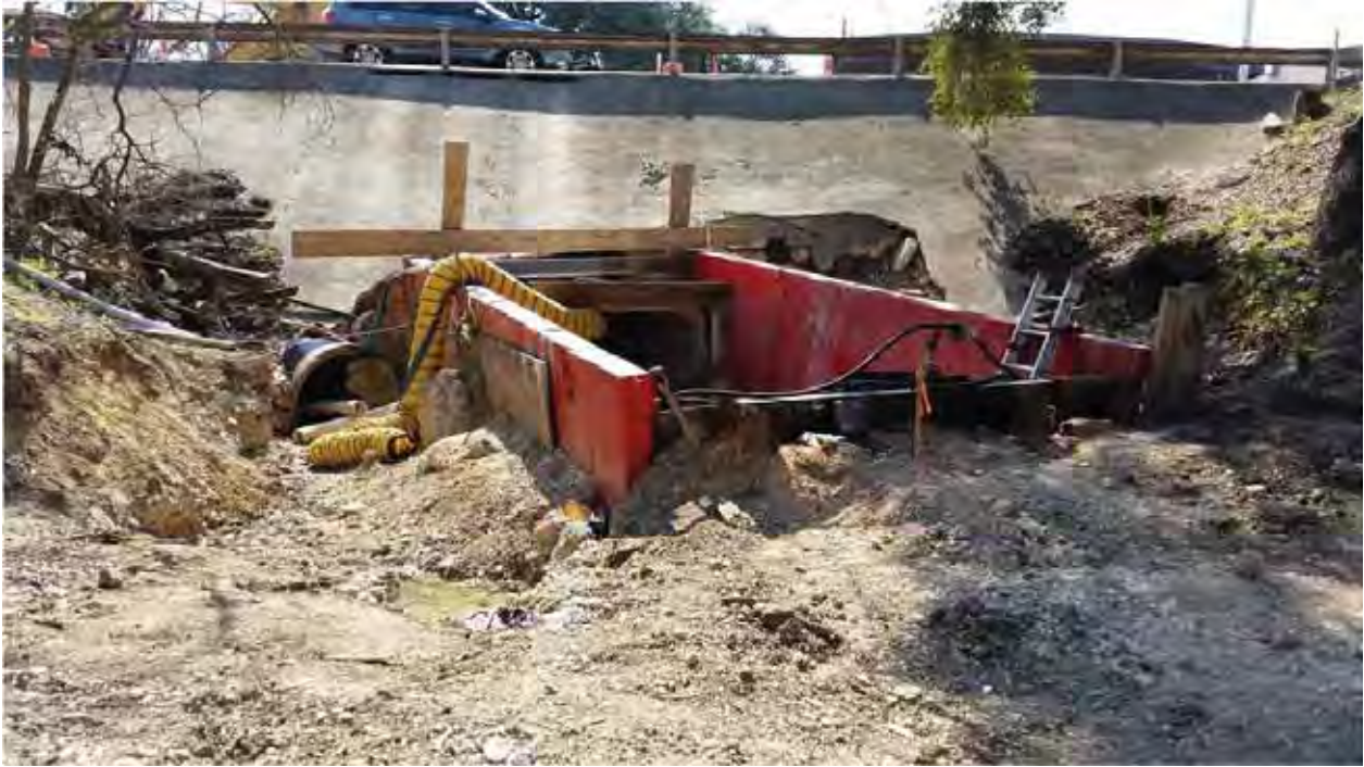
Figure 3. Exterior view of existing RCP and box culvert construction on north side of E. Court Street (looking south).
