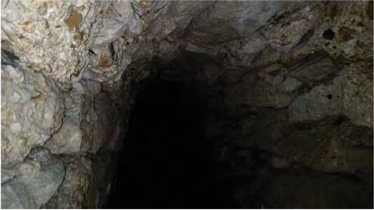
Figure 6. View of conglomerate rubble course in central portion of culvert, looking north.
