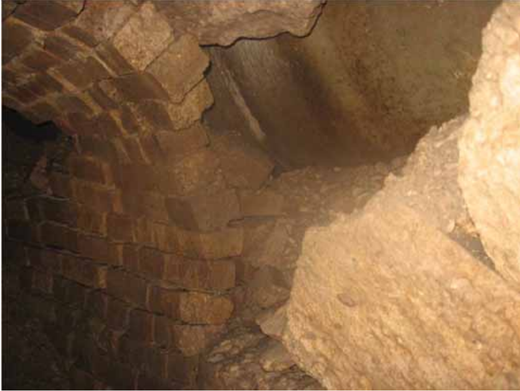
Figure 12. View of northeastern culvert segment where RCP base runs parallel to on east side.
