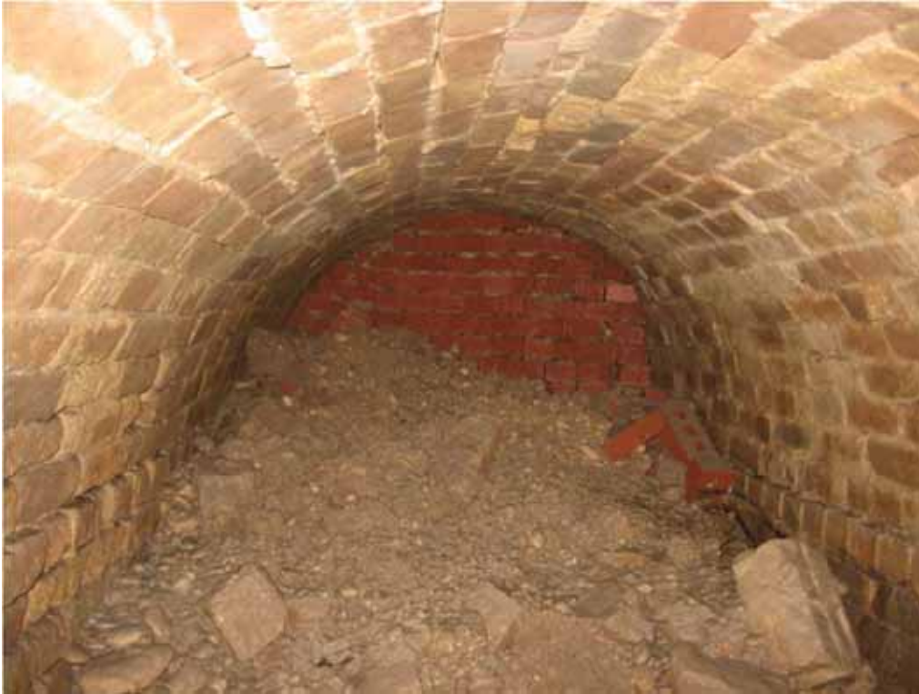
Figure 9. View of capping with modern machine-made brick at north end of culvert.
