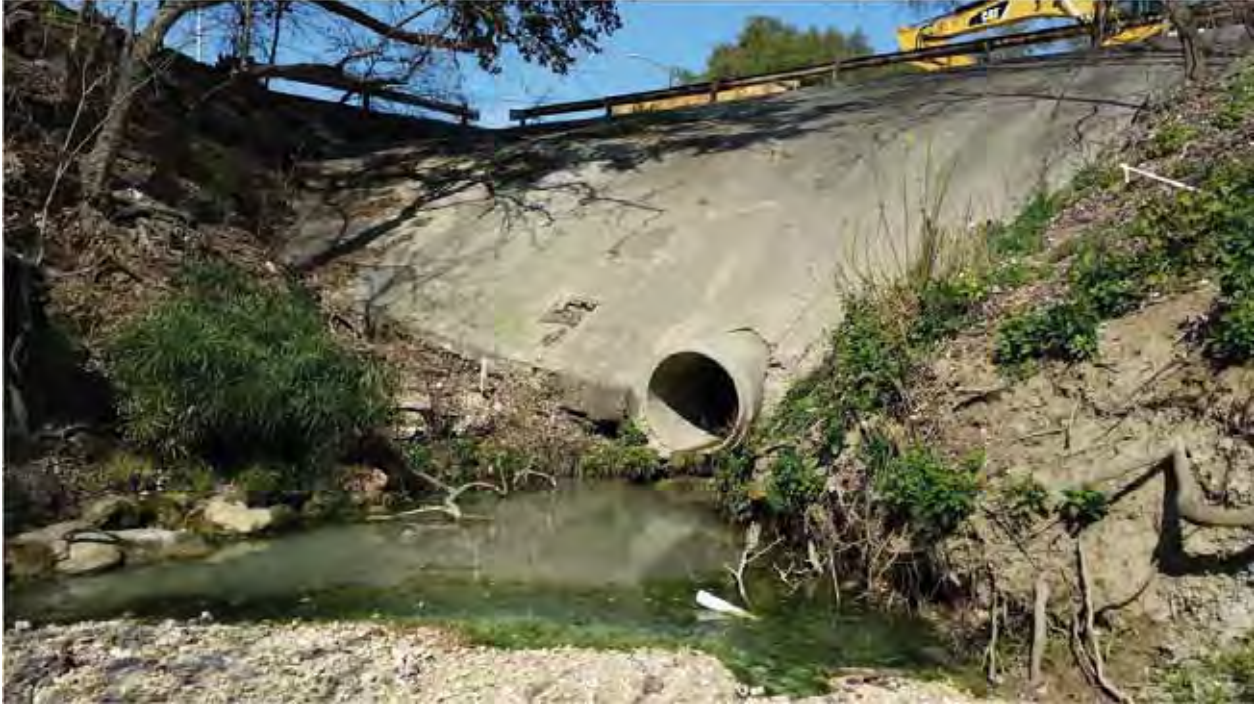
Figure 5. Exterior view of existing RCP on south side of E. Court Street (looking north).
