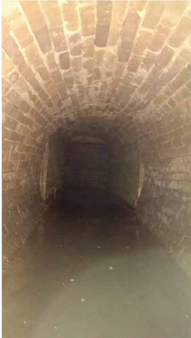
Figure 3. View of tunnel looking south illustrating transition between brick masonry walls and the cast-concrete walls of the architectural feature. Turn in tunnel visible at end of cast-concrete segment (VPS 2015).
