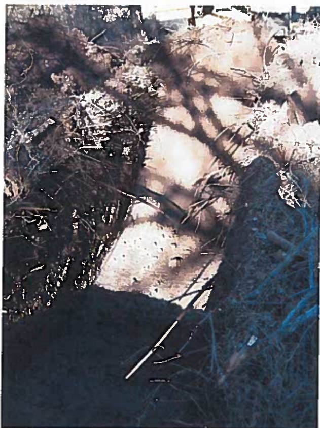
Photo 10: Facing east toward GAT #4. This trench was excavated into the east side of the creek. It was negative for archeological remains.
