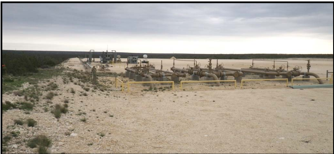
Figure 8. Photo facing northwest, proposed pump station located under southeast corner of existing station.
