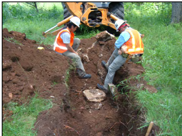
Figure 5.14. Concrete fragments, tile, and other building materials were encountered at 1 m deep in BHT 18, facing east.
