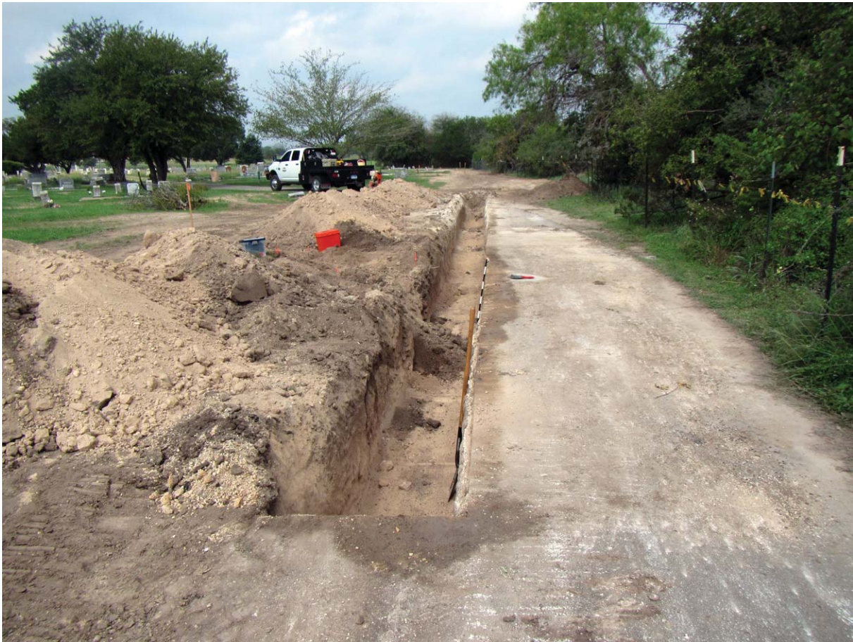
Figure 11. Photograph of the completed excavation of Trench 4, with previously excavated Trench 3 (on the left) already backfilled. View is to the northwest with the previously excavated and backfilled Trenches 1 and 2 in the background. The red-handled brush at right center marks the location of Borehole 3, and the two boxes at left center mark the heads of the two unmarked graves (the shallow scrape has also been backfilled).
