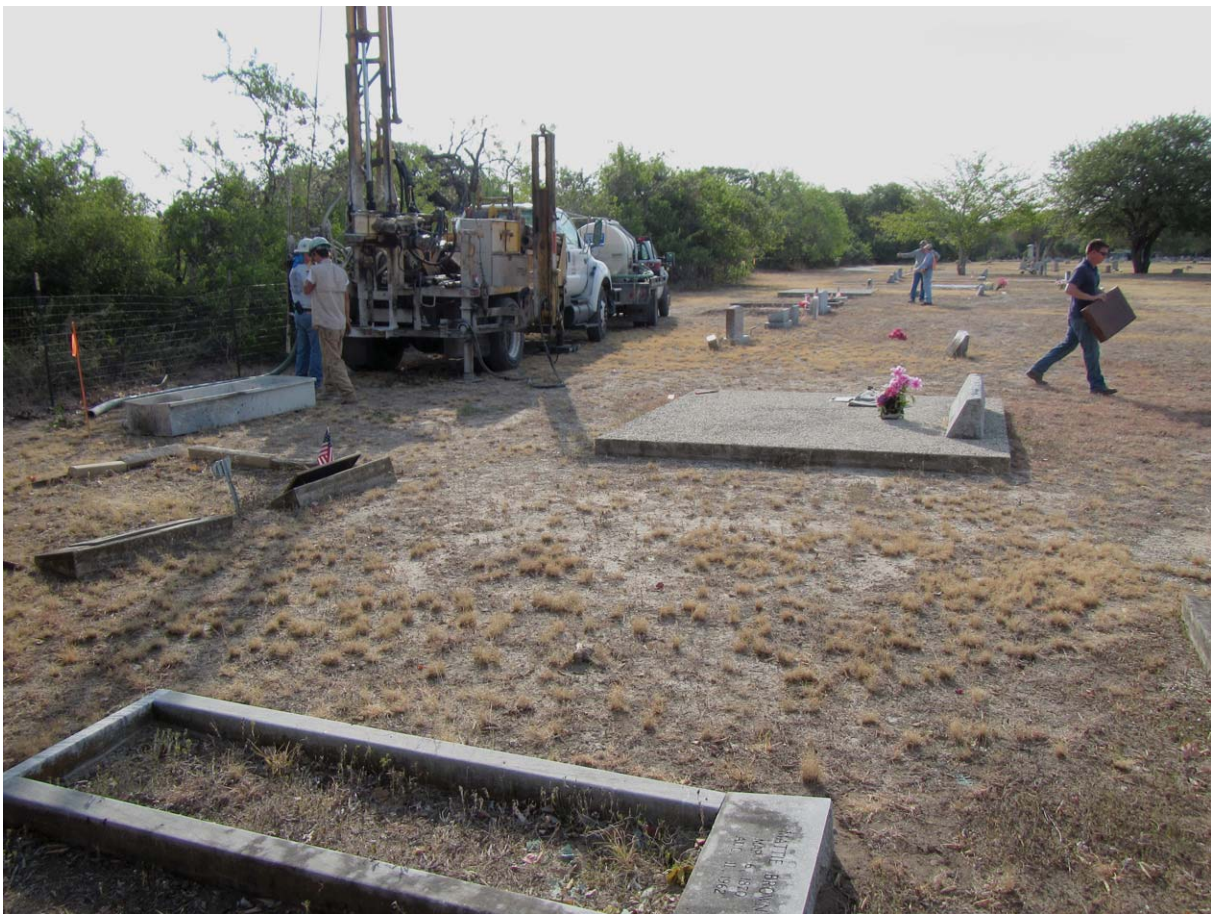
Figure 4. Photograph of the drilling in progress at Borehole 1. View is to the east, and the orange-flagged stake is the baseline mapping point 10 + 00 ft. Note the proximity of the marked graves.
