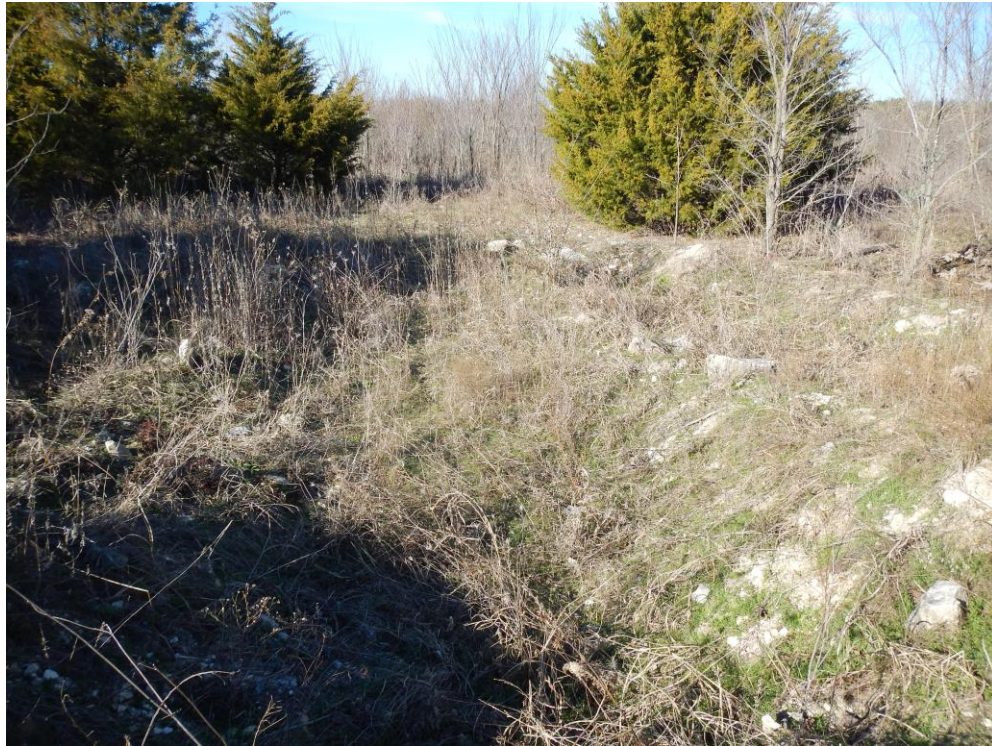
Figure 15. Large scour made by heavy equipment; facing northwest. Note bedrock slabs on walls and surface.
