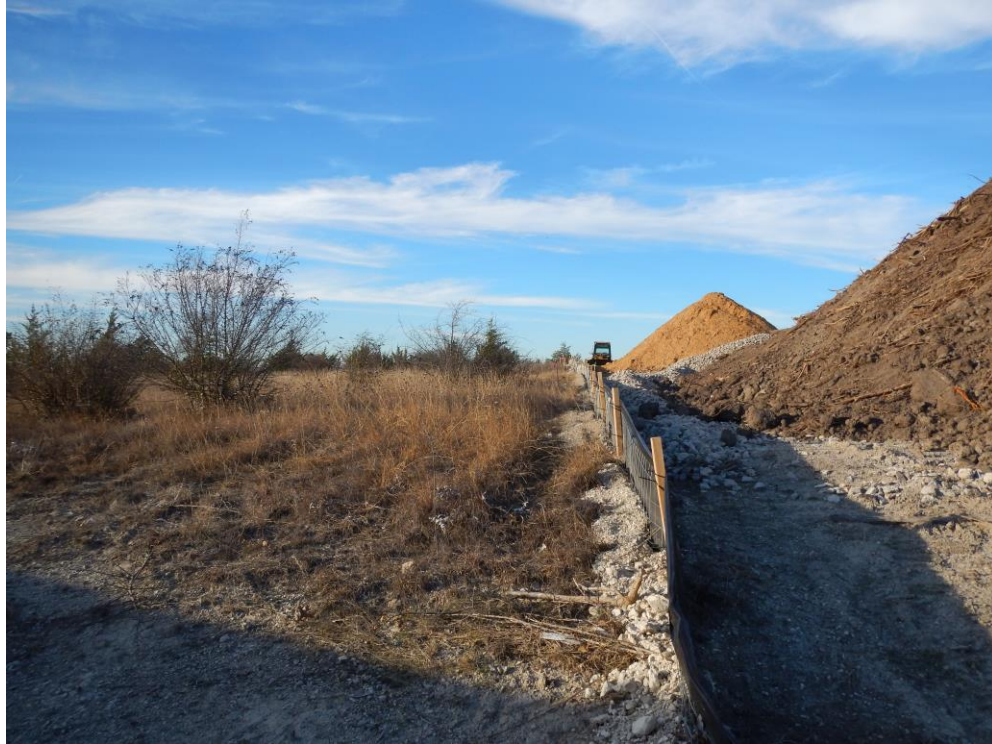
Figure 3. View along the east boundary with DART construction on right; facing northwest
