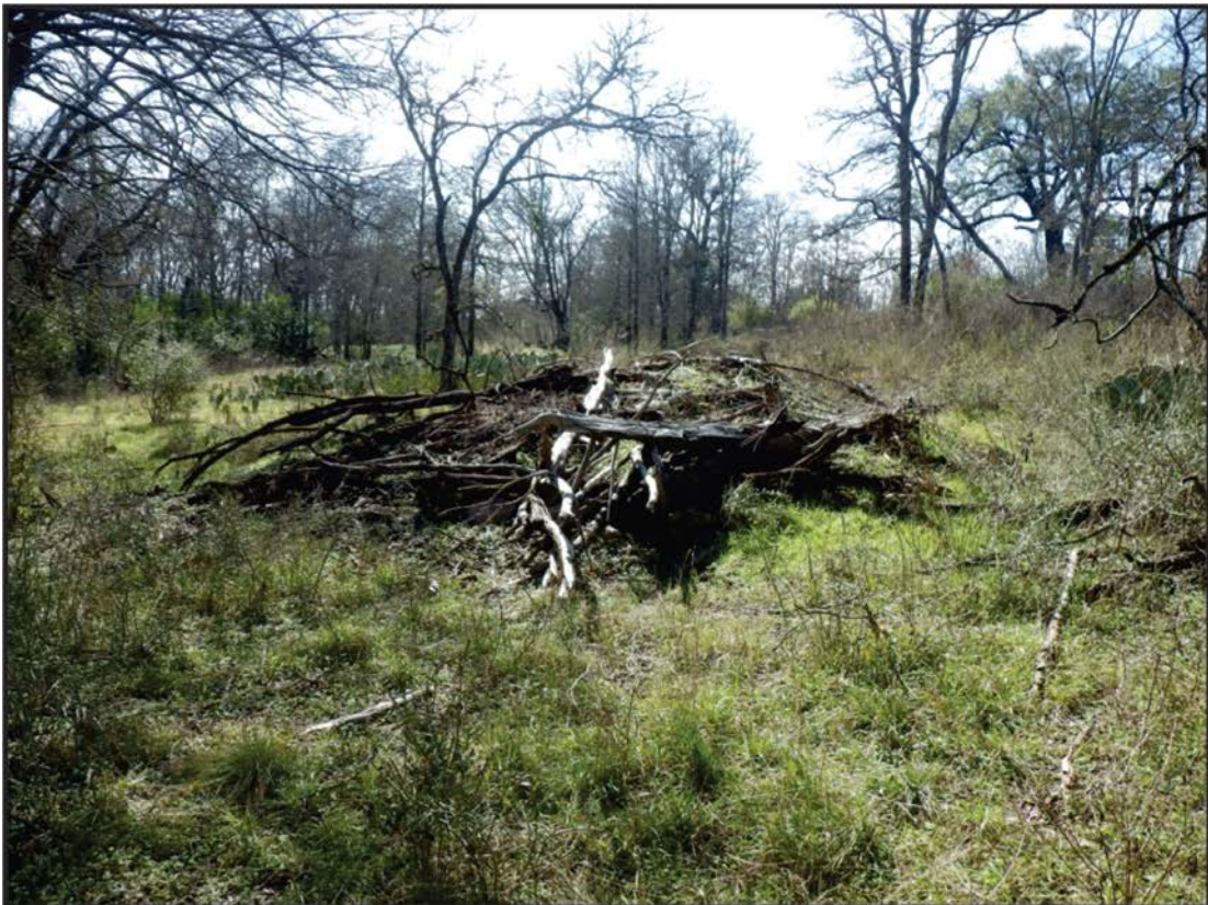
Figure 5. Terrace bench clearing looking south at typical brush pile and pushed rock pile.
