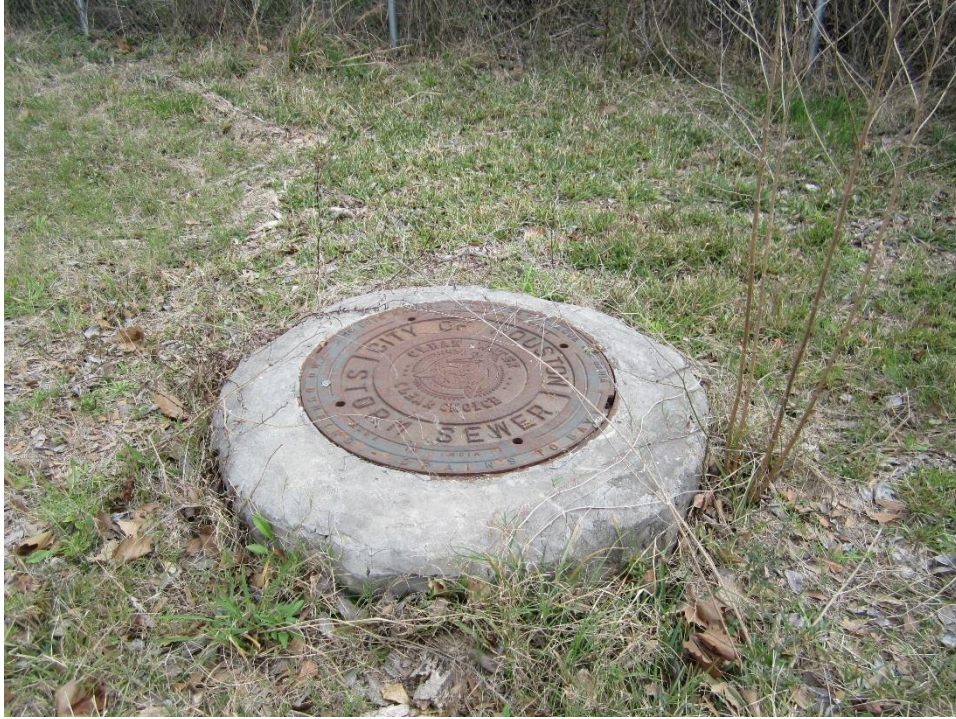
Figure 5-6. Sewer manhole at right angle turn of proposed hike and bike trail corridor on Mercer Arboretum property.
