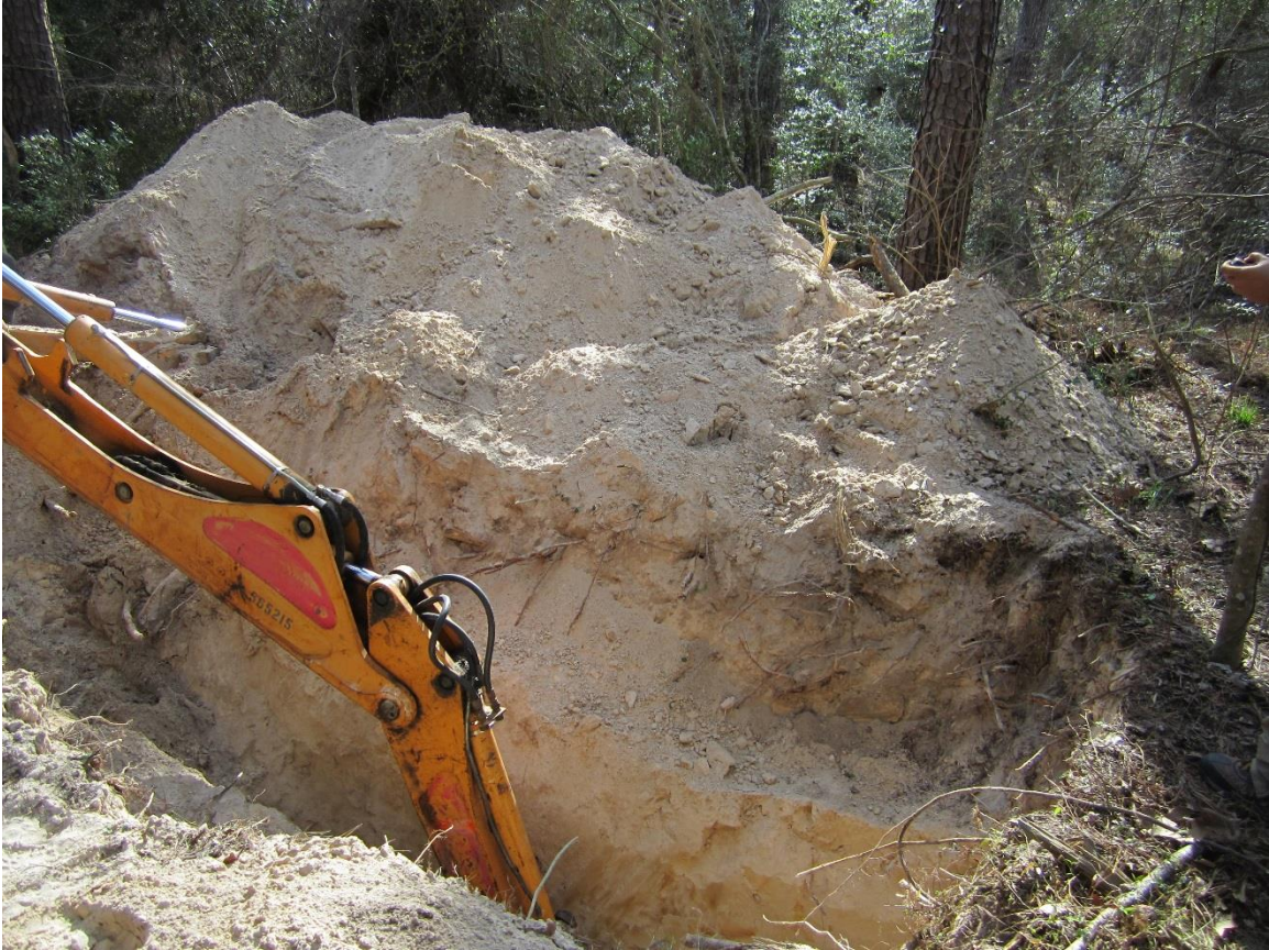
Figure 5-12. Last phase of excavation in progress at Trench 1, removing soil to reach 12 ft.
