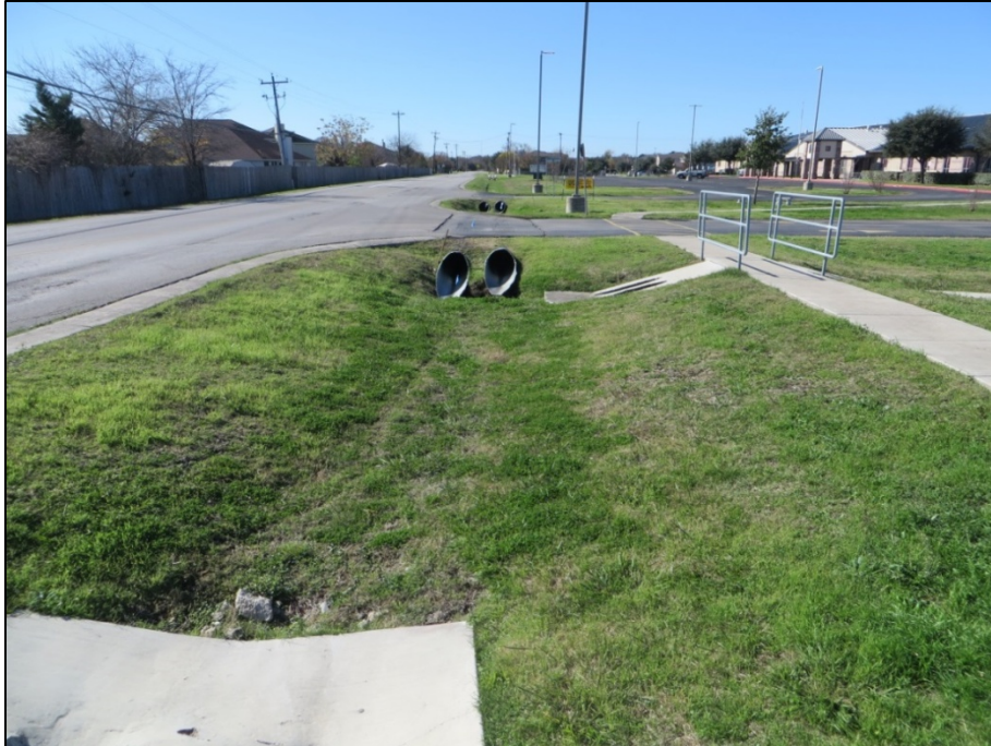
Figure 1-4. West side of the ROW facing southwest. Note drainage ditch, culverts and driveways.
