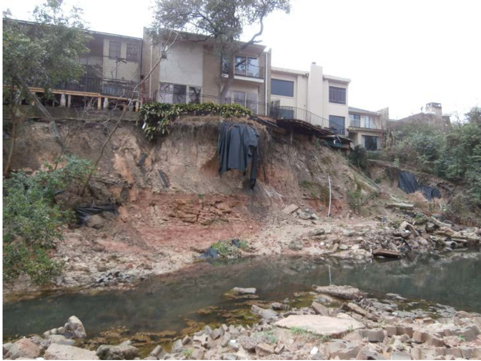
Figure 5. Eroded bank of Spring Branch channel, with failed bank stabilizing debris.
