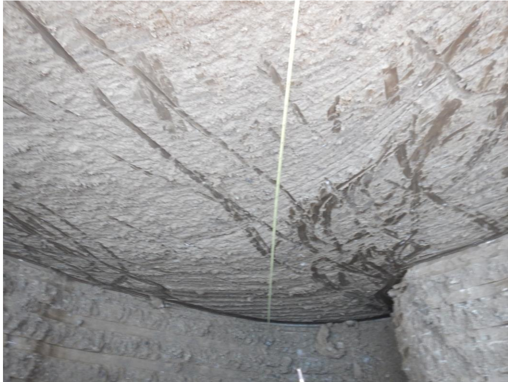
Figure 10. Bottom of south wall profile in Trench 2. Note water seep at bottom of Trench 2.
