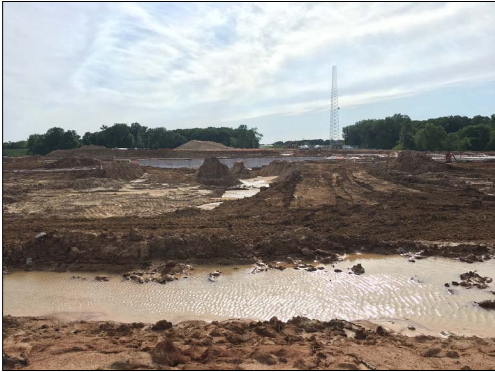
Figure 8. Overview of pump station construction from the point of the peninsula (facing west).
