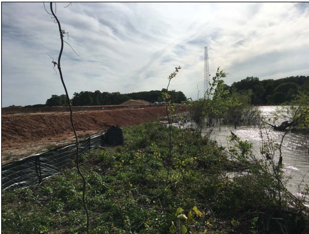
Figure 6. View of pump station construction from a small undisturbed portion of 41HE377 on the north side of the peninsula (facing west).
