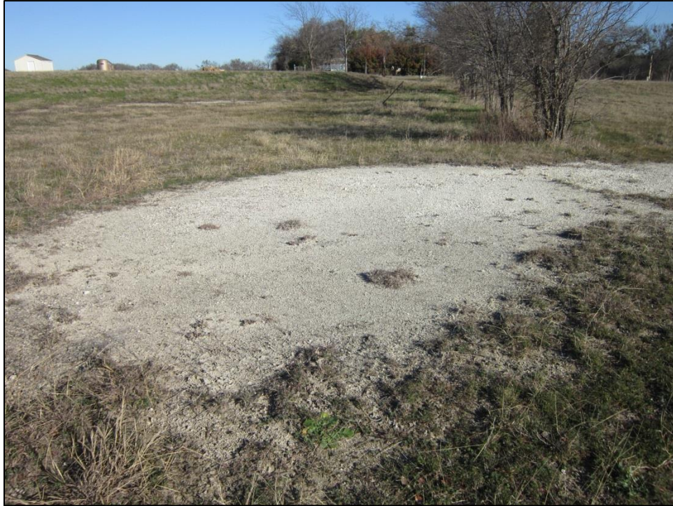
Figure 15. Eroded soil with exposed bedrock as seen within disturbed auxiliary spillway. Facing west.
