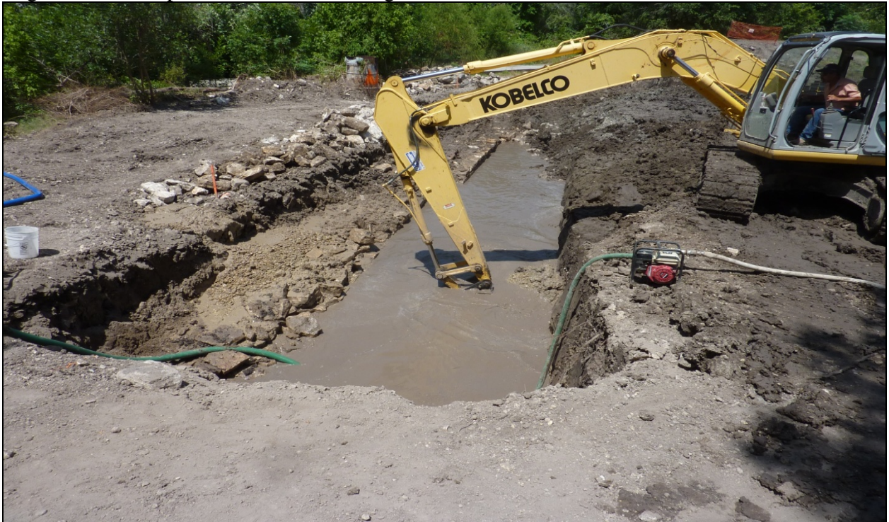
Figure 3. Deep trenching operation for the new dam wall. Note the old historic dam wall to the left of the trench and remnant walls at the edge of the water.
