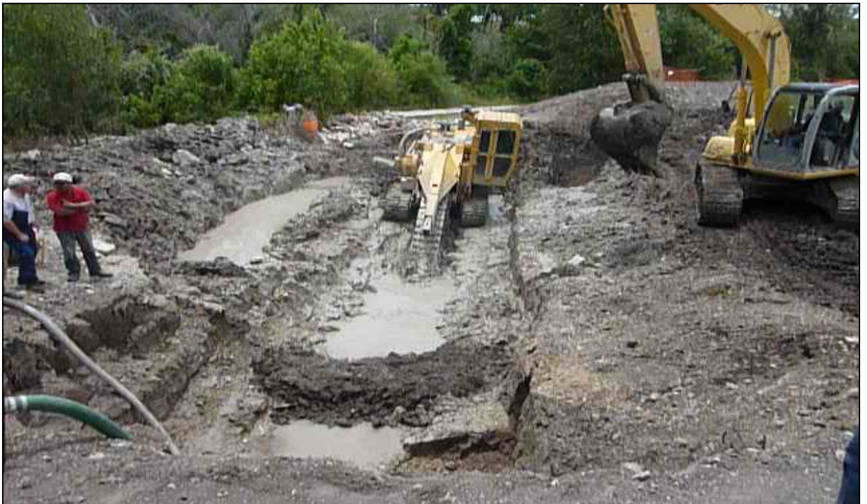
Figure 5. Trenching down into bedrock, original historic dam wall at left of trenching machine, in the mud.
