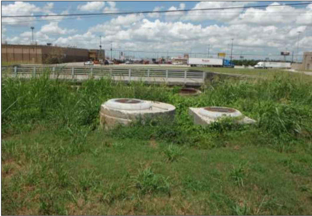
Figure 8. Storm Water Manholes Located at Northern End of Project Area, Facing West
