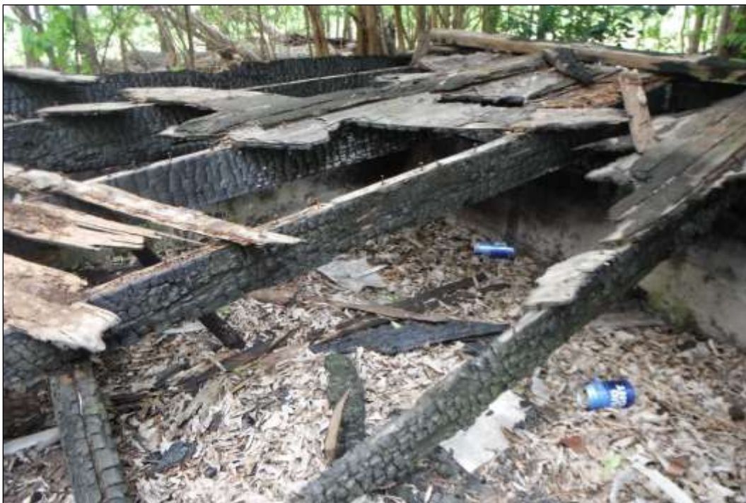
Figure 6-64. Structure W6-A (41HY541)—Remnants of Burned Frame on Eastern Outer Porch (Facing East)
