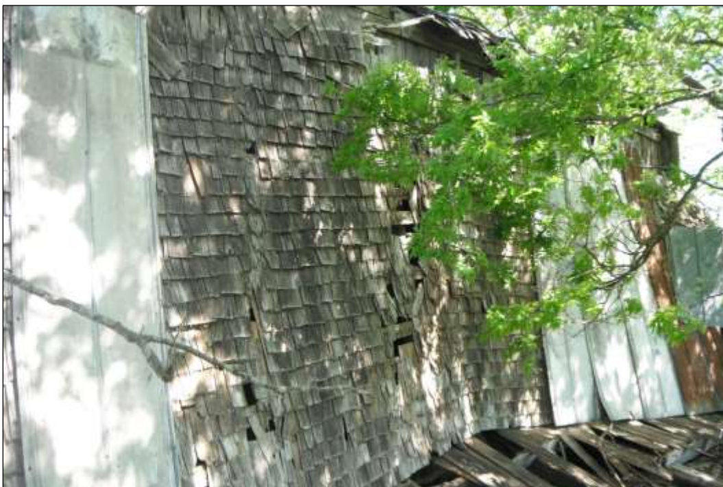
Figure 6-46. Resource 2—Collapsed Porch Roof on Southern (Front) Façade of House (Facing Northeast)
