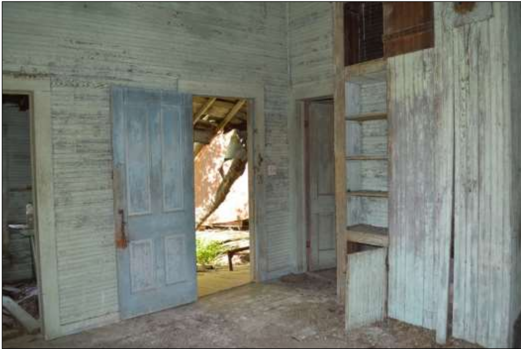
Figure 6-19. Resource 1A—View of Kitchen and Door Leading to Southern Porch (Facing Southwest)
