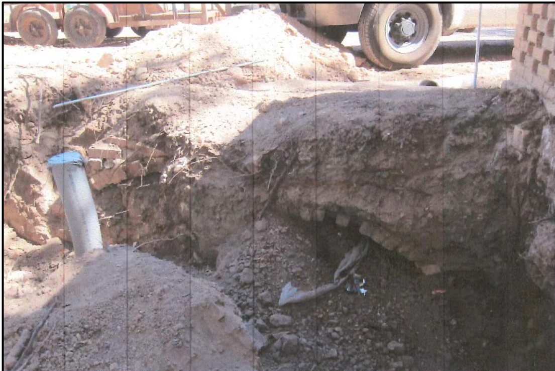
Figure 4-5. Original excavations of Cistern 2 in February, 2016. Note the two arches of the cistern and the parking lot in the background.
