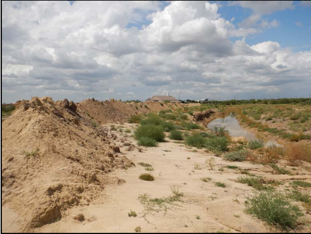
Figure 8. Augmented drainage channel crossed by proposed APE (see Figure 9-3 for location where photograph was taken).
