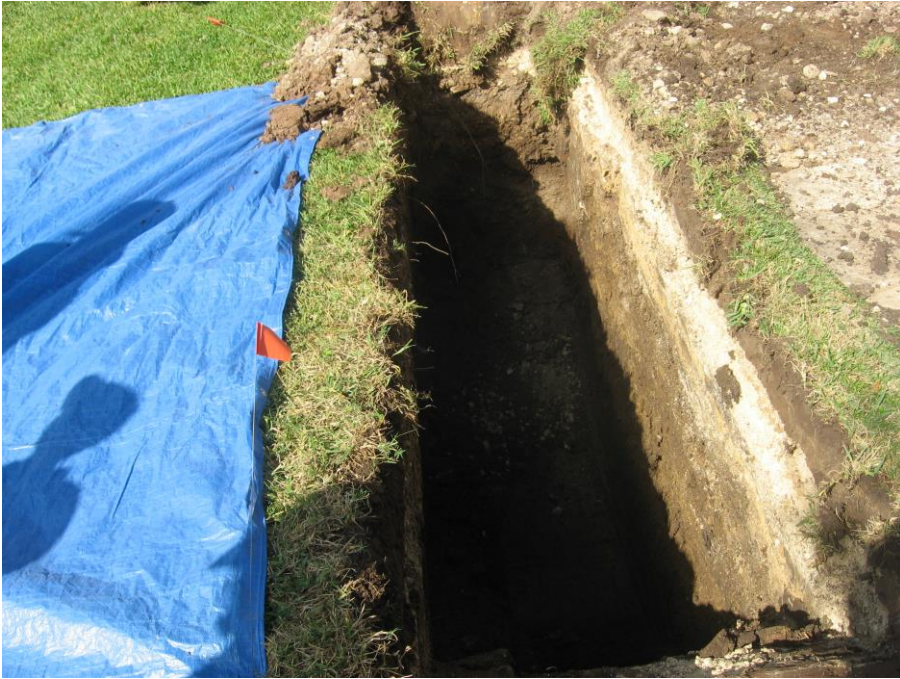
Photo #4: Facing west toward Gradall Trench (GT) #1. Note the fill levels in the right hand side of the frame.
