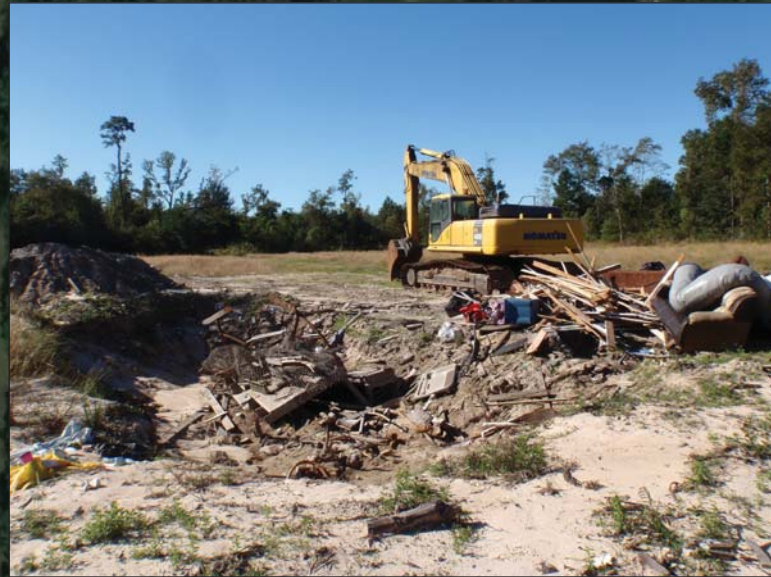
A. Modern trash dump. View is to the southwest.
