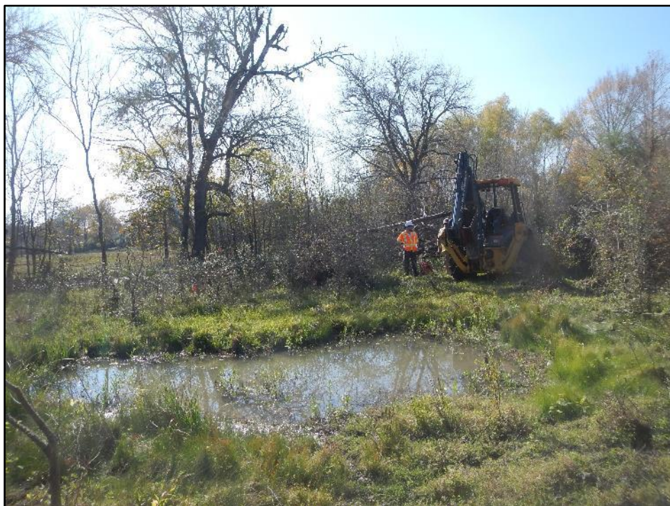
Figure 7. Overview of APE along low-lying floodplain of East Mill Creek, facing southeast.
