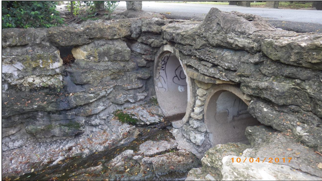
Figure 19. Close-up of where culvert and retaining walls meet. Only the culvert portion will be replaced (41TR306).
