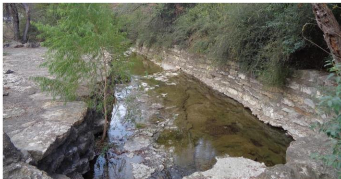
Figure 7: View of stone-lined creek banks from on top of the culvert. Looking east.
