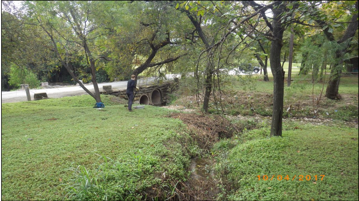
Figure 9. Overview of the Culvert Replacement survey area, ST11 and site 41TR306. View is to the southeast.
