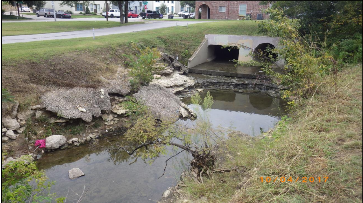
Figure 11. Looking at Zoo Creek north of the modern culvert on McPherson Ave. View is to the southeast.
