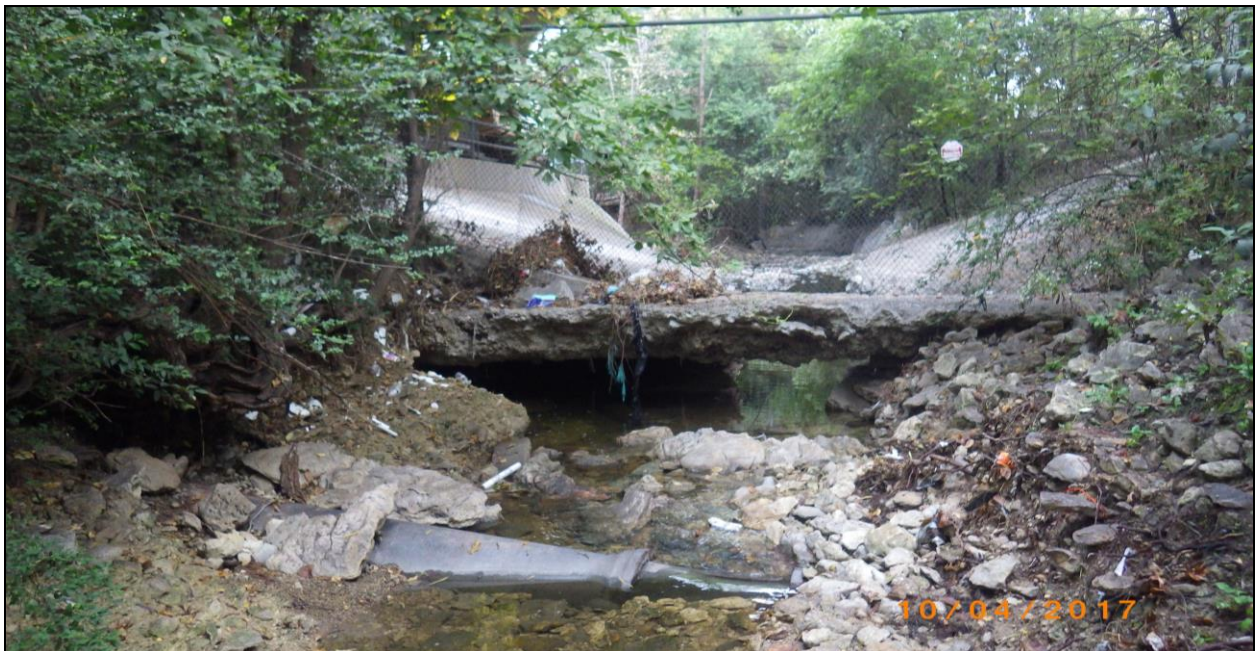
Figure 7. Exposed sewer line in Zoo Creek under Park Hill Bridge.
