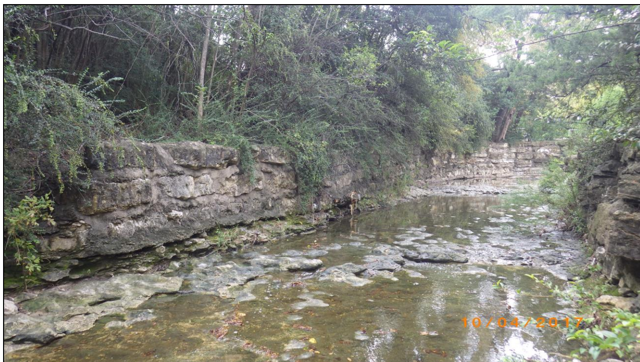
Figure 18. Retaining walls on the downstream (east side) of culvert (41TR306). View is to the southwest.
