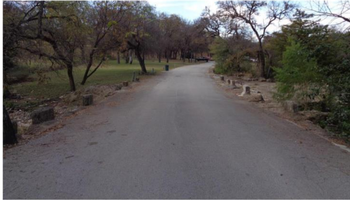
Figure 4: View north up South Forest Drive as it crosses the Forest Drive/Zoo Creek Culvert.
