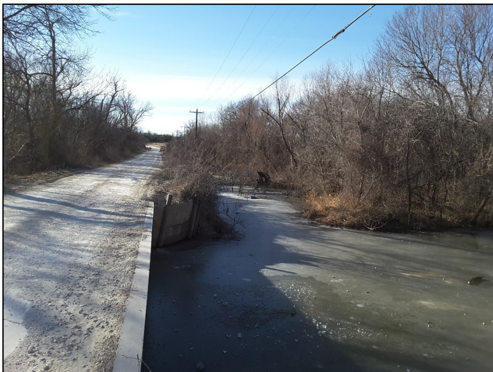
Figure 6. Overview of bridge and Herring Branch crossing showing inundated areas within APE, facing south.
