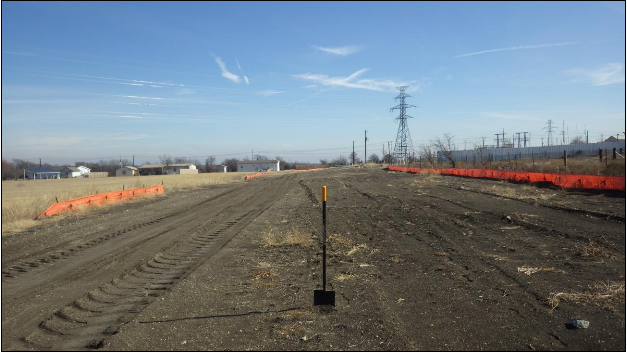
Figure 9. Construction disturbance within survey route, ST26-27 were not excavated. View is facing east.
