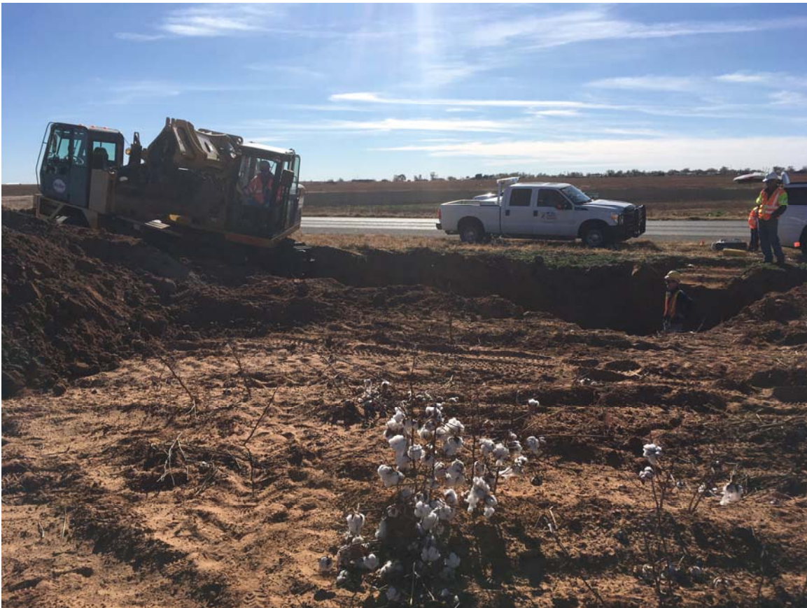
Figure 10: View of scraping in progress. Note orange pin flag on far right of frame, which marks location of road-parallel buried utility. For a different perspective, see Figure 7.
