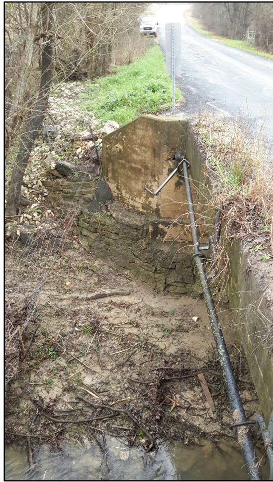
Figure 6. Boyce Lane bridge spanning Harris branch, eastern side of road facing south.
