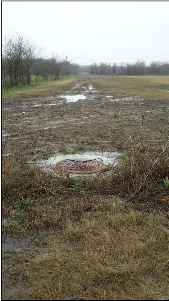
Figure 8. Recently installed wastewater line on northern end of project area, facing west.
