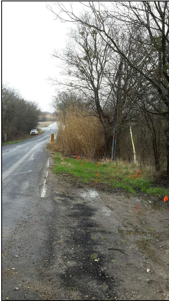
Figure 7. Multiple marked utilities near Harris Branch on western side, facing south.
