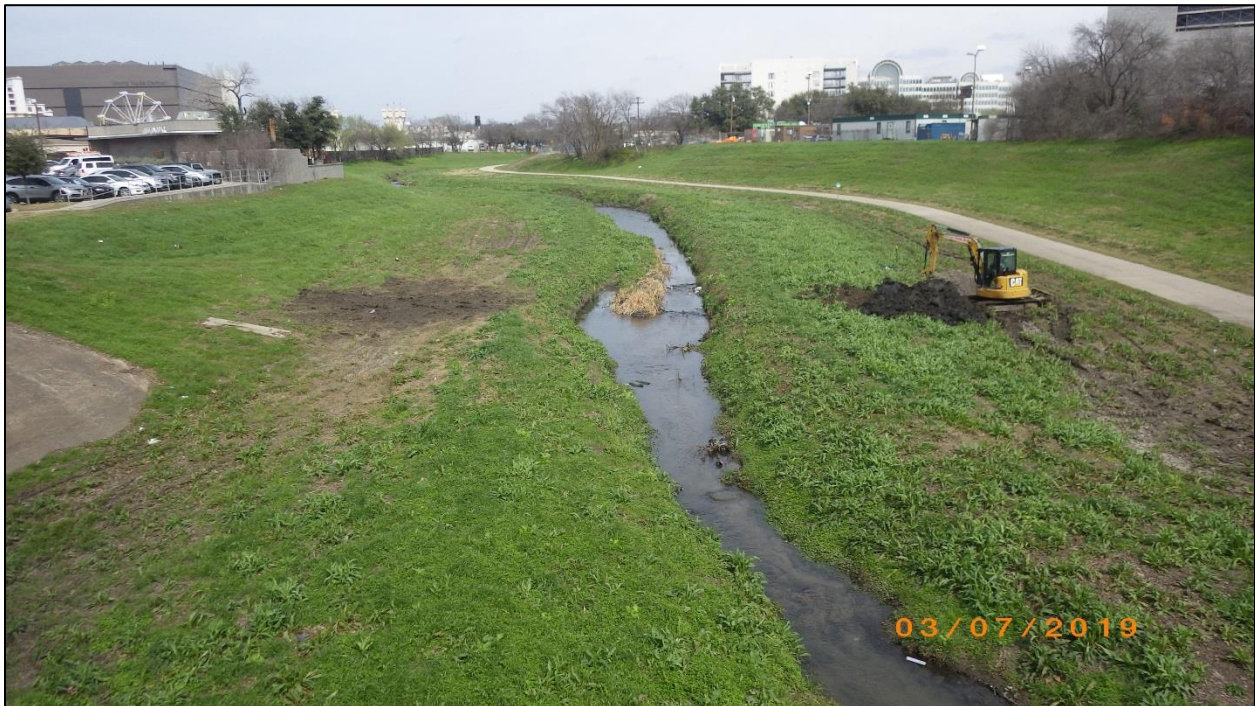
Figure 2. DWU 84-Inch Wastewater Main project overview. The east (right in the photo) channel bank is approximately 30 cm higher than the west (left in the photo) channel bank.
