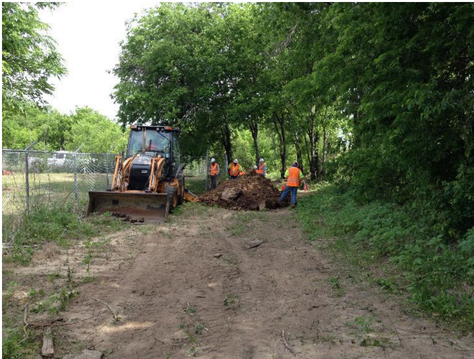
Figure 6. Overview of northern project area with BHT D under excavation. Facing north.
