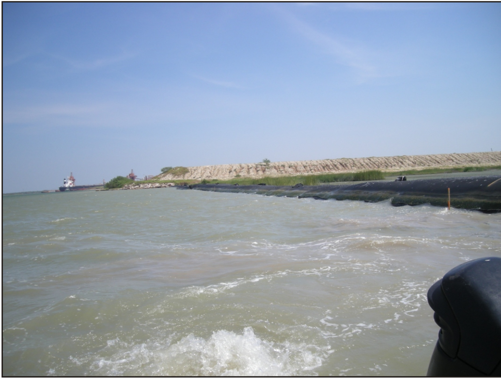
Plate 1. North running fabric erosion barrier leading to concrete and rebar shore protection at the base of a dredge spoil deposition area.
