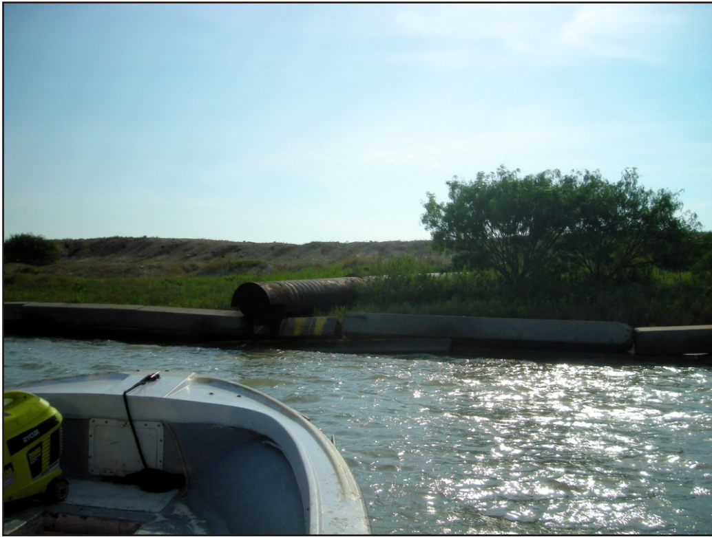
Plate 3. Detail of dredge spoil pipe line to move dredged materials into spoil containment area.
