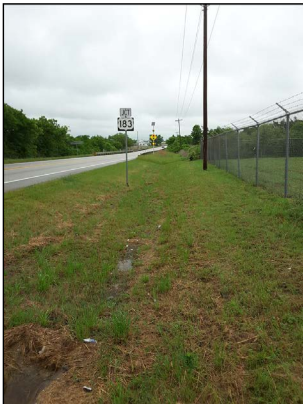
Figure 8. Overview of approach along FM 1625 to bridge spanning North Fork Dry Creek, facing northwest.
