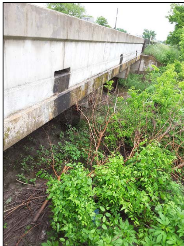
Figure 9. Overview of FM 1625 bridge at North Fork Dry Creek, drainage, and pilings; facing northwest.
