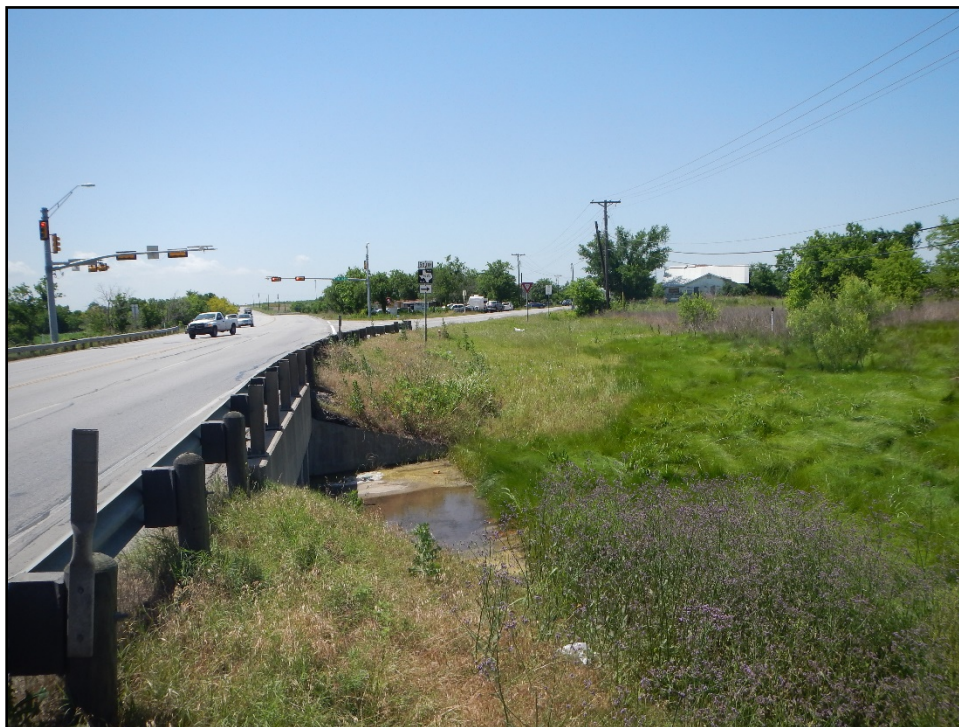
Figure 10. Overview of US 183 bridge at the tributary of North Fork Dry Creek and project area, facing south.
