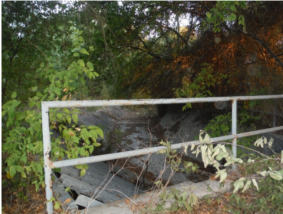
Figure 13. Concrete channel near Hypothesized Acequia Lateral A west of Espada Road, facing north.
