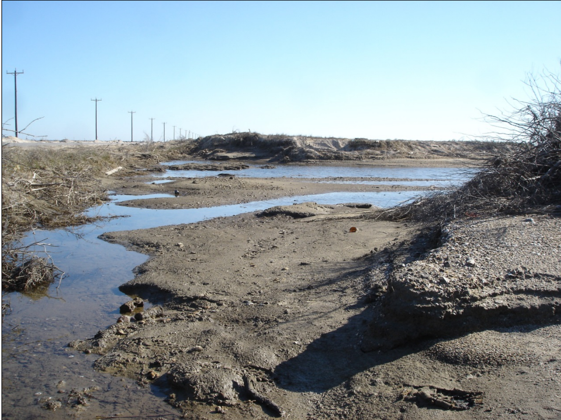
Figure 8: Illustration of backbeach scour adjacent to US87 roadway.
