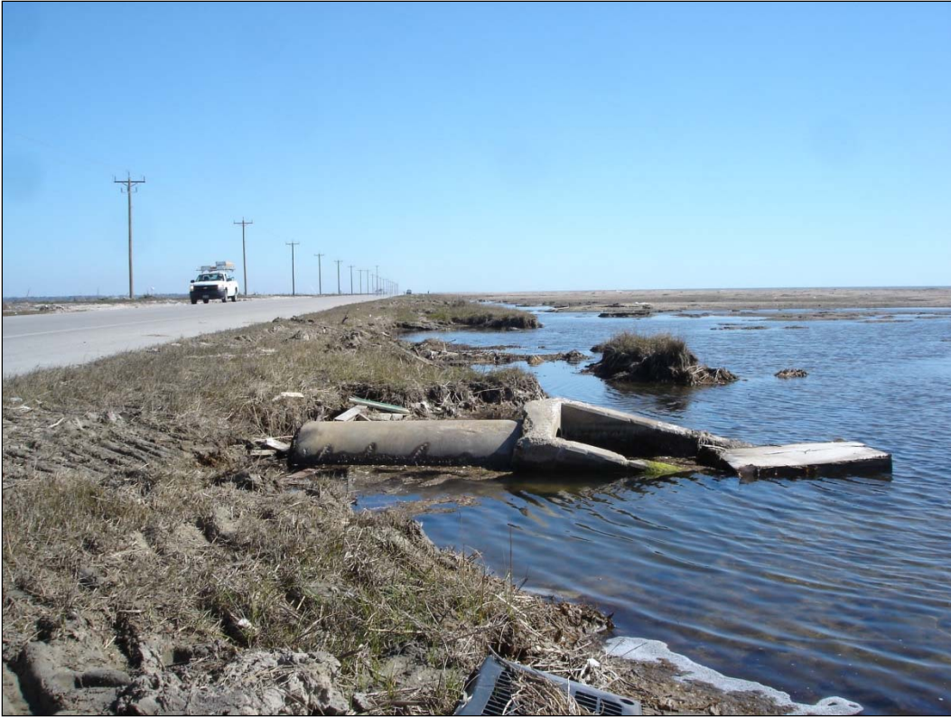
Figure 9: Exposed, safety-end-treated concrete culvert illustrating erosion in the US87 ROW.
