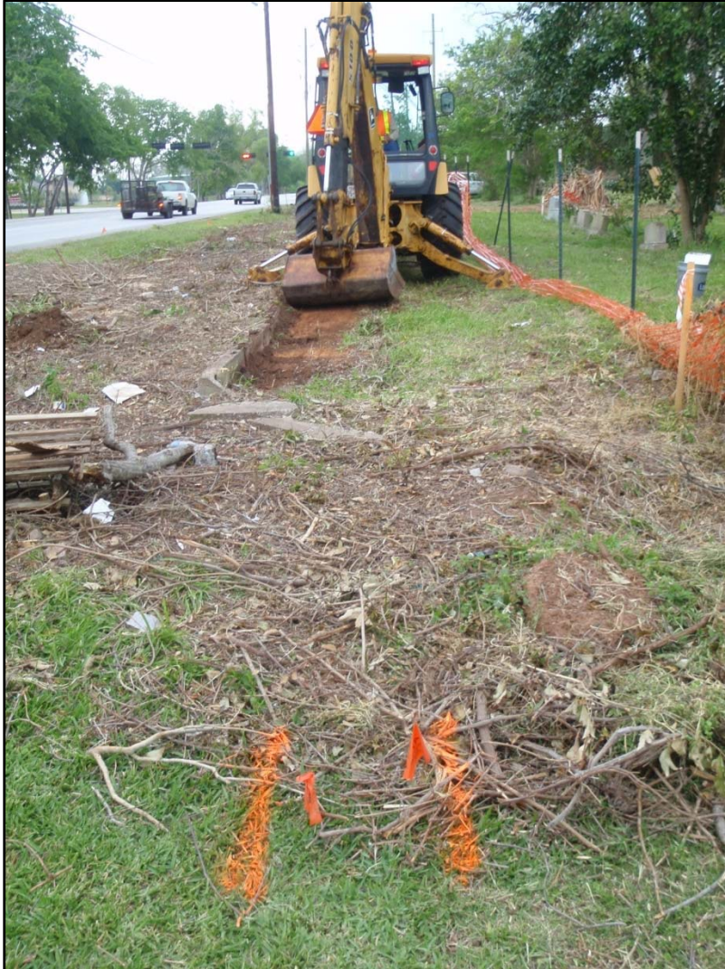
Figure 10: View of backhoe initiating scraping in existing ROW in front of New Home Cemetery.
