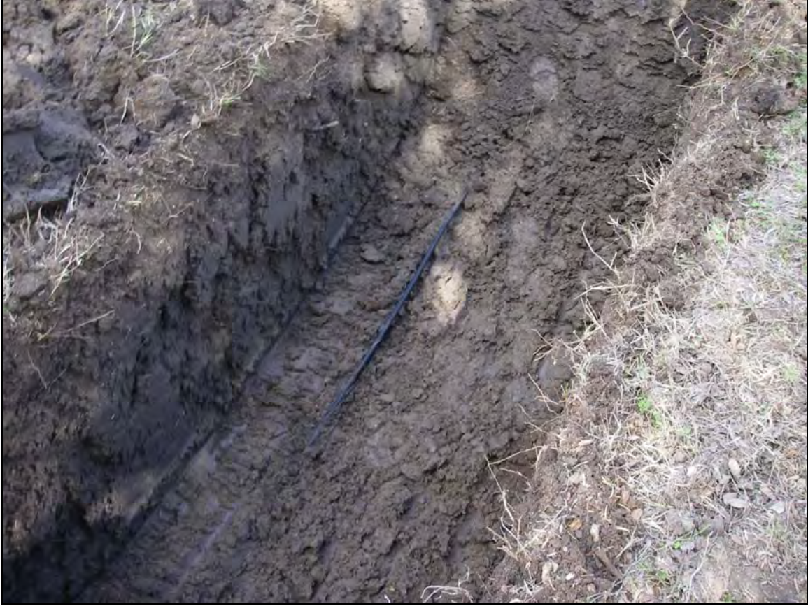
Figure 7. Exposed unmarked buried utility in BHT 3 north of the northern Peck-Bush Road at San Miguel Creek crossing.
